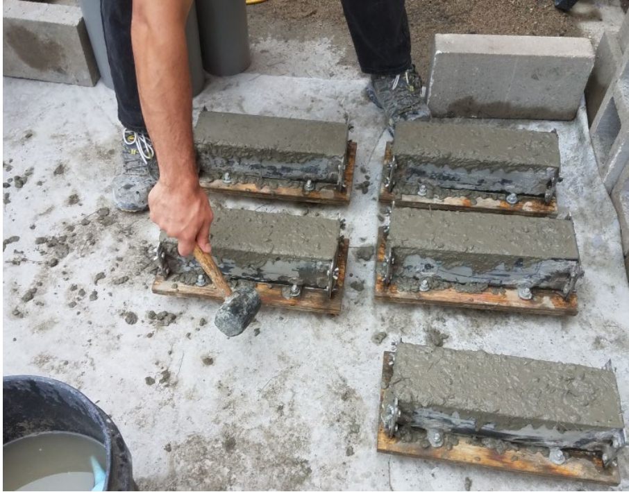
Figure 3.5 Use of rubber mallet to obtain final consolidation efforts of the concrete
