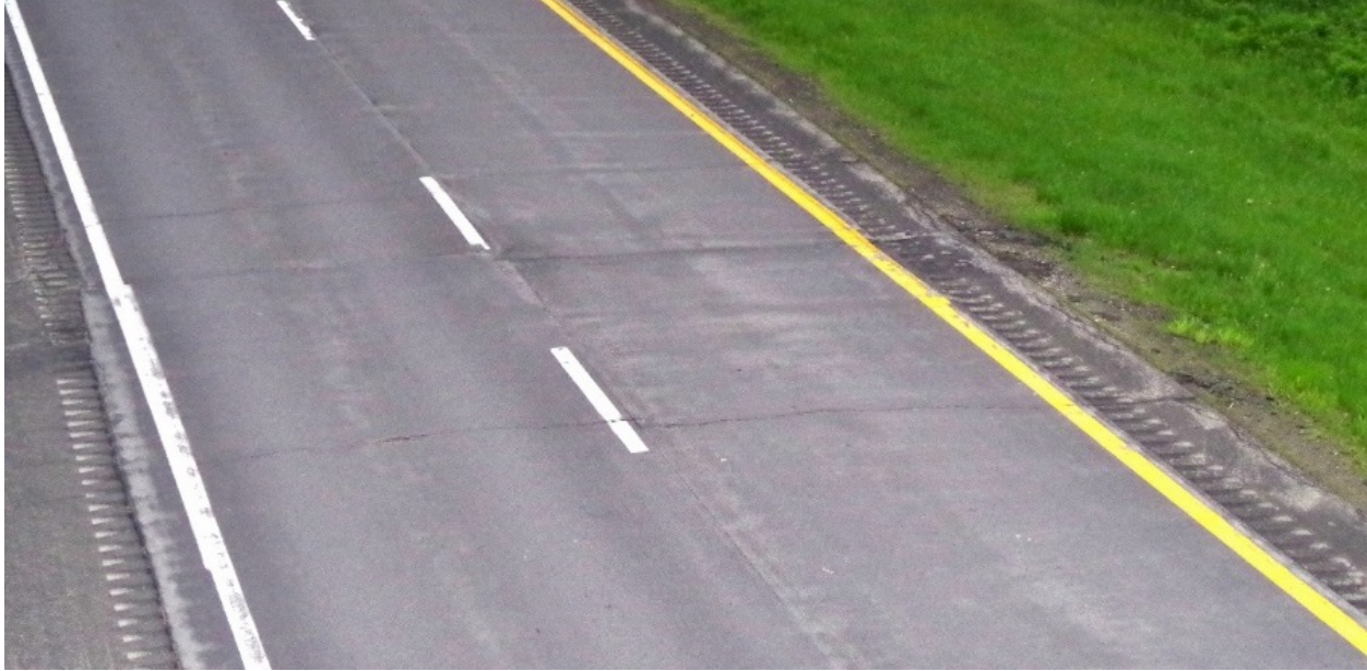
Figure 67: Photo. Cracks above the concrete joints in 2015.
