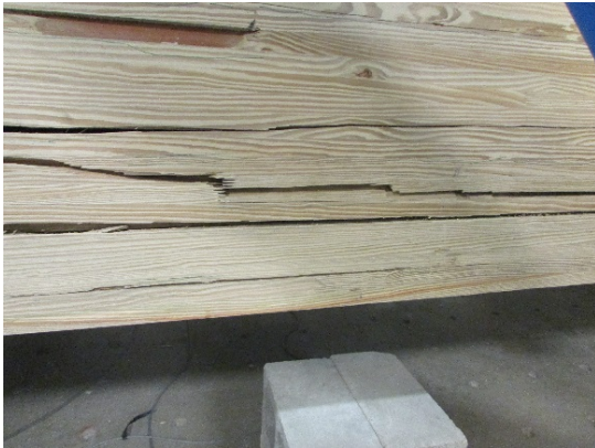
(a) Failure of West Girder
