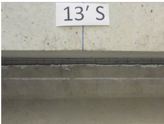
(c) Shrinkage Cracks in Haunch Region of Girder B Filled with Non-Shrink Grout
