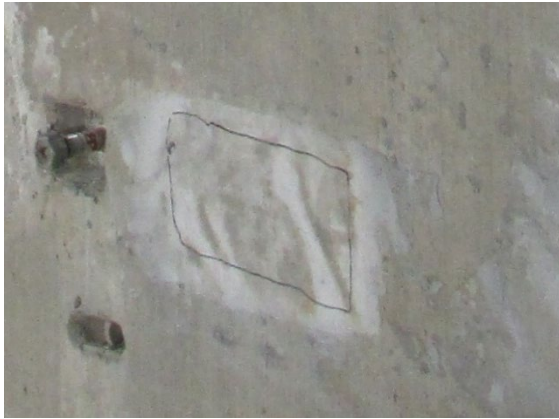
(a) Non-Shrink Grout at 125,000 Cycle
