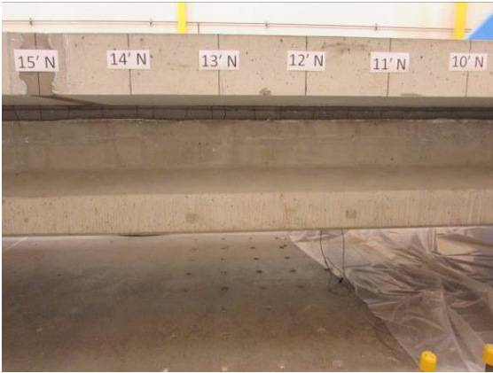
(a) Shrinkage Cracks in Haunch Region of Girder A Filled with Latex Modified Concrete
