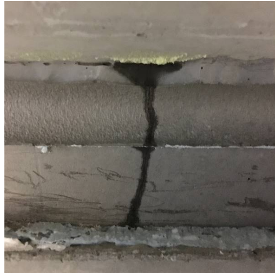
(b) Close Up of Crack
