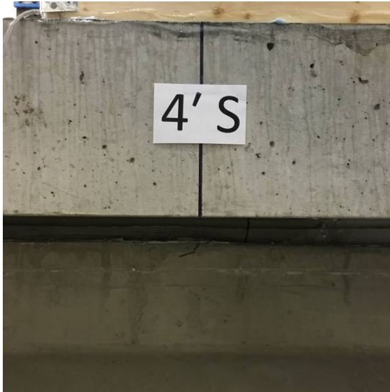
(a) Observed Crack at 25,000-Load Cycle
