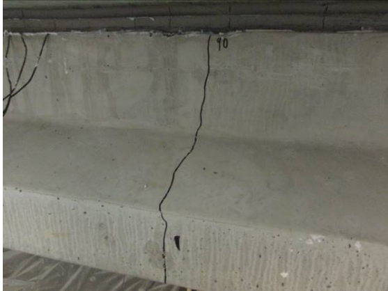
(a) First Crack, Mid-Span of Girder A at P = 251 kips
