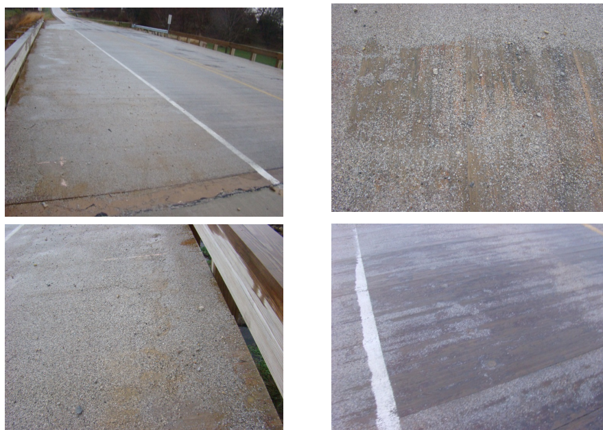
Figure 3.29 Epoxy with Embedded Grit Wearing Surface for Glulam Timber Bridge in Buchanan County, Iowa
