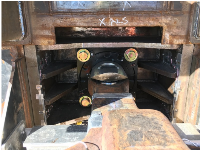
Figure 34. PBC installed within the sliding lug
