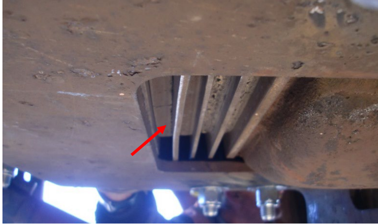
Figure 14. M1 bent buff plate in draft gear
