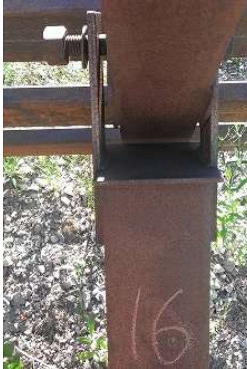
Figure 65 Strut connection with nut almost off of bolt
