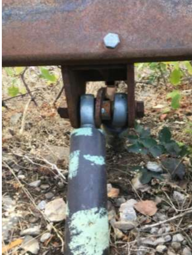
Figure 63 Example of epoxy paint missing on foundation connection couplers
