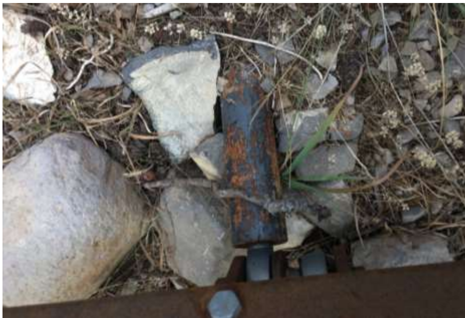
Figure 62 Example of corrosion on micropile foundation coupler without epoxy paint
