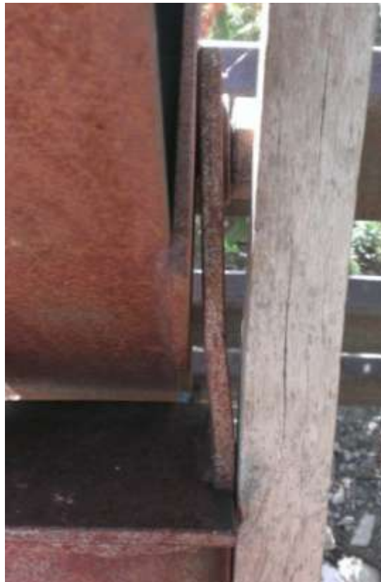
Figure 66 Deformation of strut-to-girder connecting plate due to over-tightening of bolt on SSS #1
