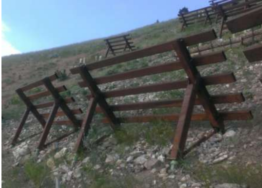
Figure 61 Row of SSS at upper region of starting zone; SSS chosen for instrumentation is at left side of photo
