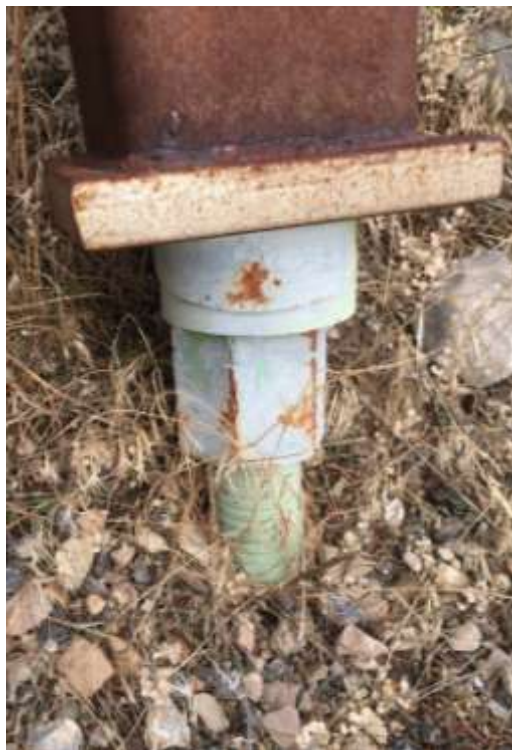
Figure 64 Chipped epoxy paint on strut foundation nut and washers
