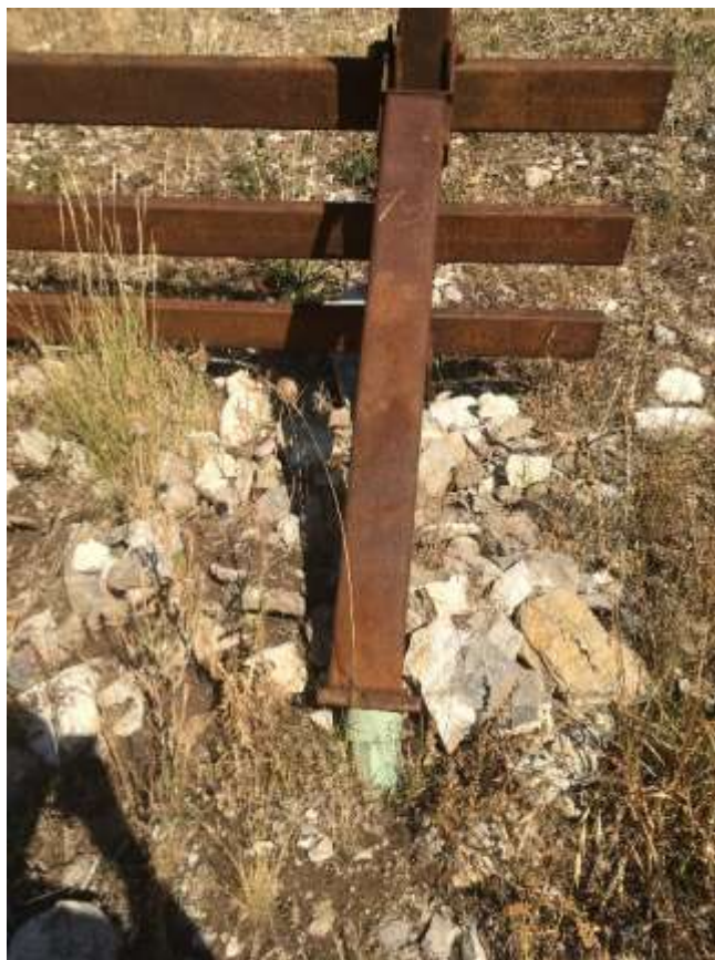
Figure 67 Misalignment of strut axis and micropile axis on structure #73
