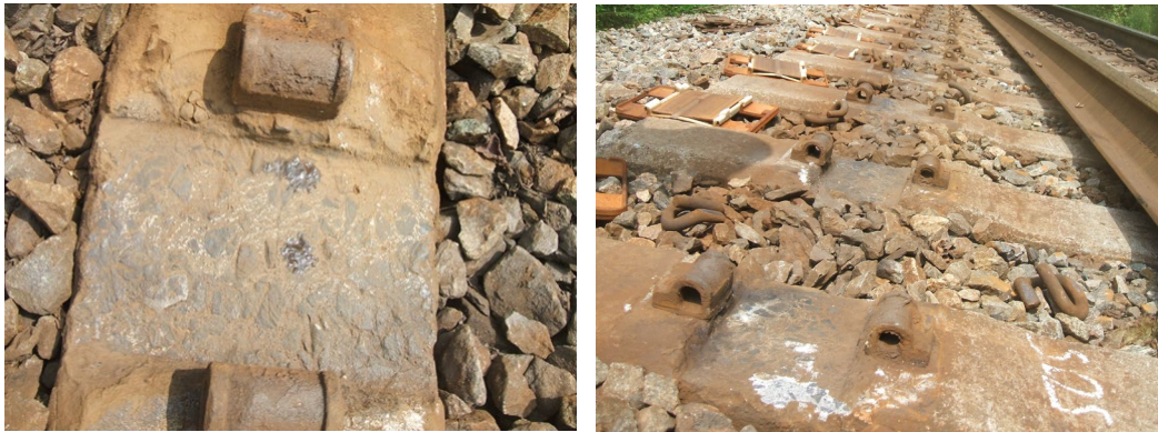
Figure 1. Rail Seat Deterioration
