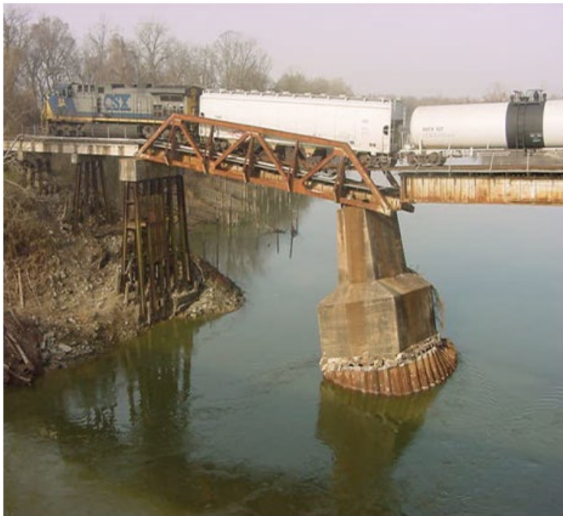
Figure 1 – Bridge Failure due to Scour
