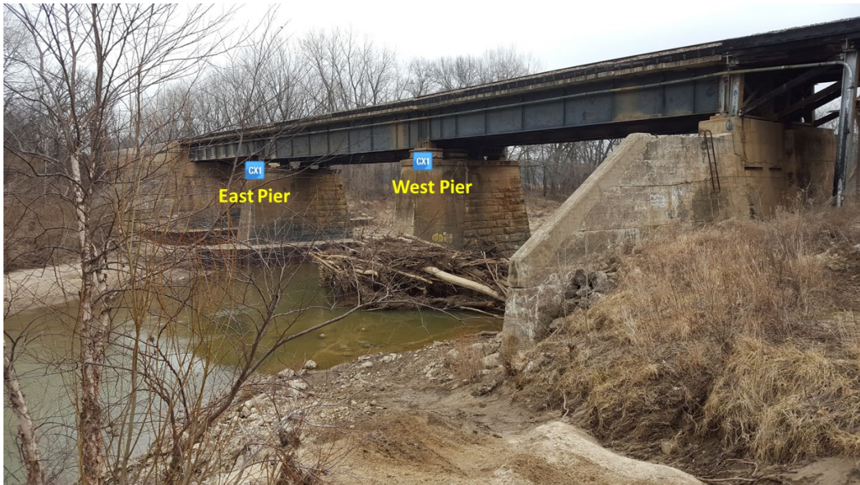
Figure 37 – BNSF Bridge 279.7 Sensor Locations
