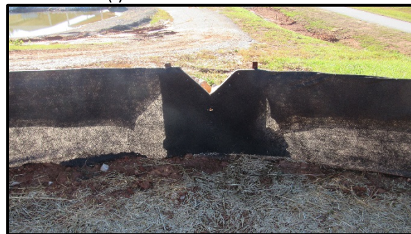
(h) field installation - upstream
