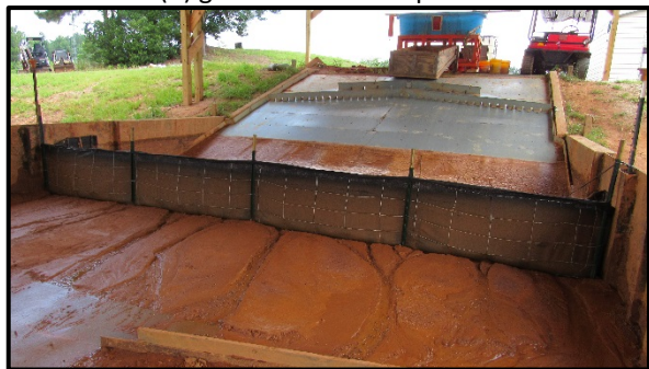
(f) M8 downstream erosion
