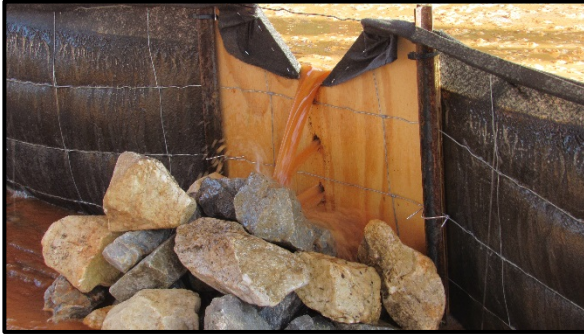
(c) riprap energy dissipater
