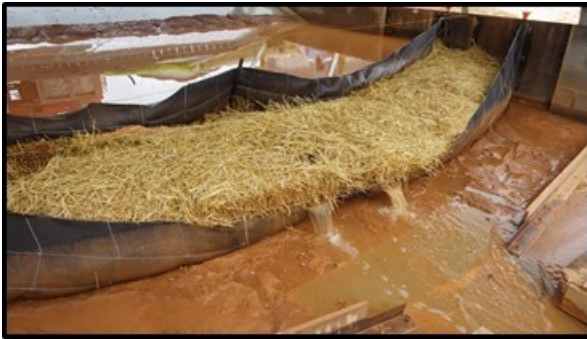
(a) ALDOT SRB overtopping
