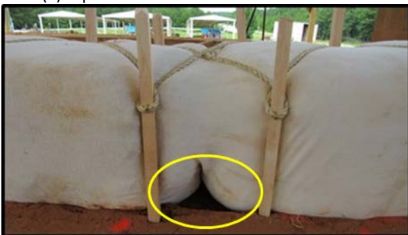
(g) rounded end abutment void
