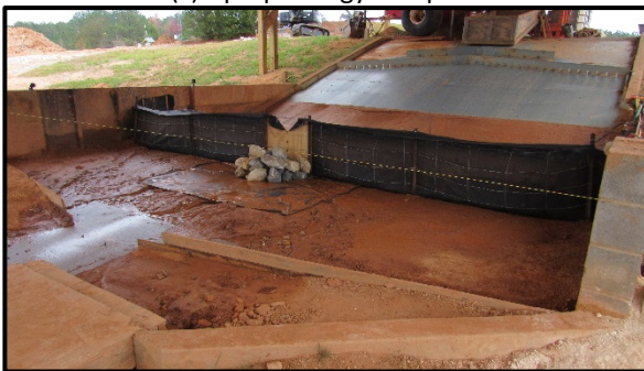
(e) M9 downstream erosion
