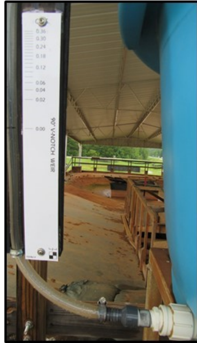
(e) flow rate monitoring
