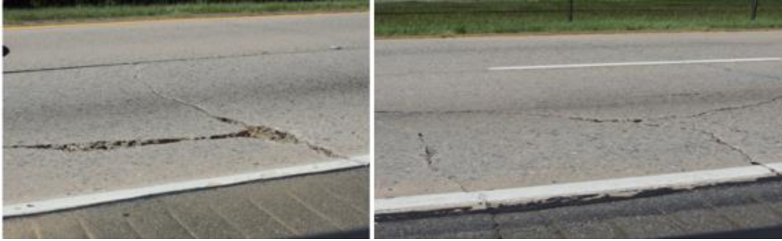
Figure 2.6 Examples of shattered slab
