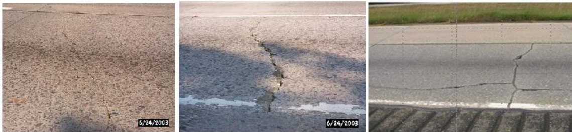
Figure 2.4 Various broken slab severity level 2
