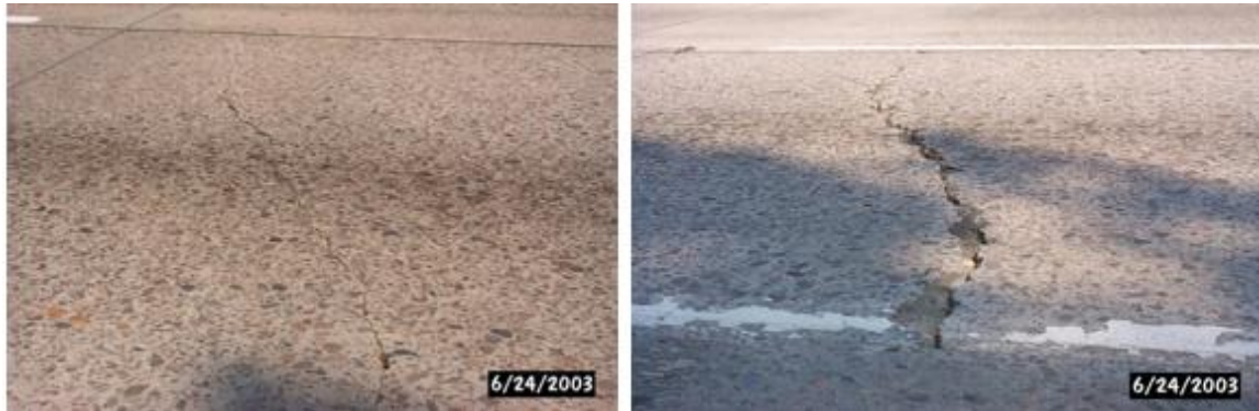
Figure 2.8 Examples of transverse cracking Severity Levels 1 and 2
