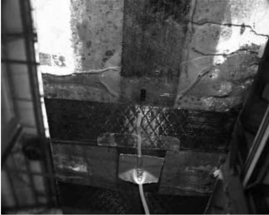
Figure 8.7 Bottom View of Specimen A-F4 Showing the Formation of Secondary Cracks during Cycling in the Vicinity of the Crack Initiator
