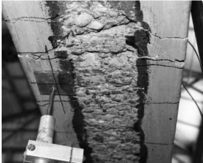
Figure 6.5 Bottom View of Specimen B1 Showing the Surface of the Concrete in the Area where CFRP Debonding Initiated
