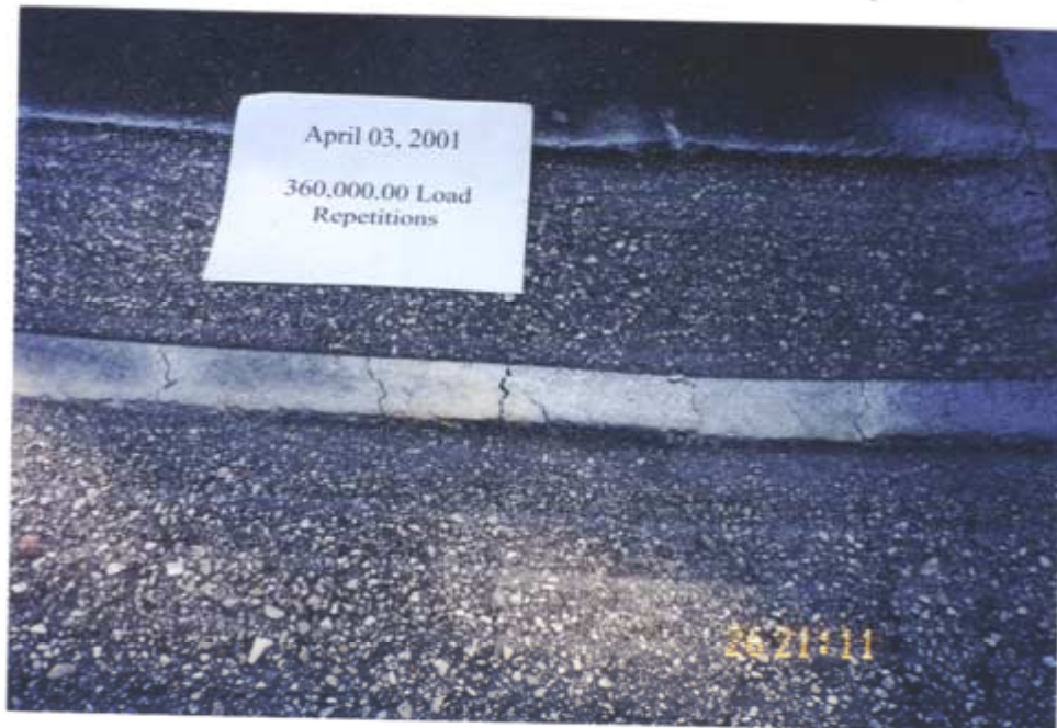
Photograph 5.20 The Transverse Cracks on the Limerock Test Section.
