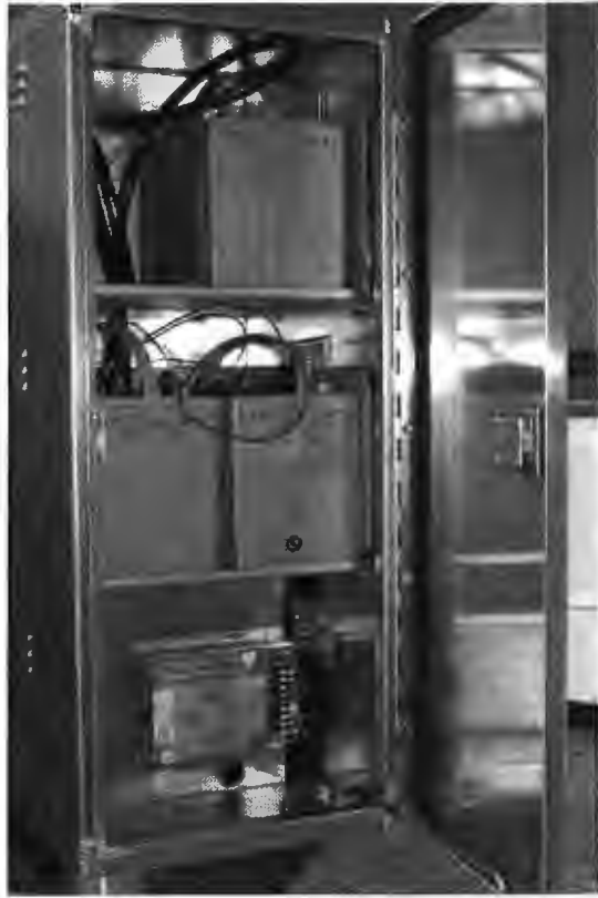
Figure 7. Power Unit Used for Tests 417920-3 and 417920-4.
