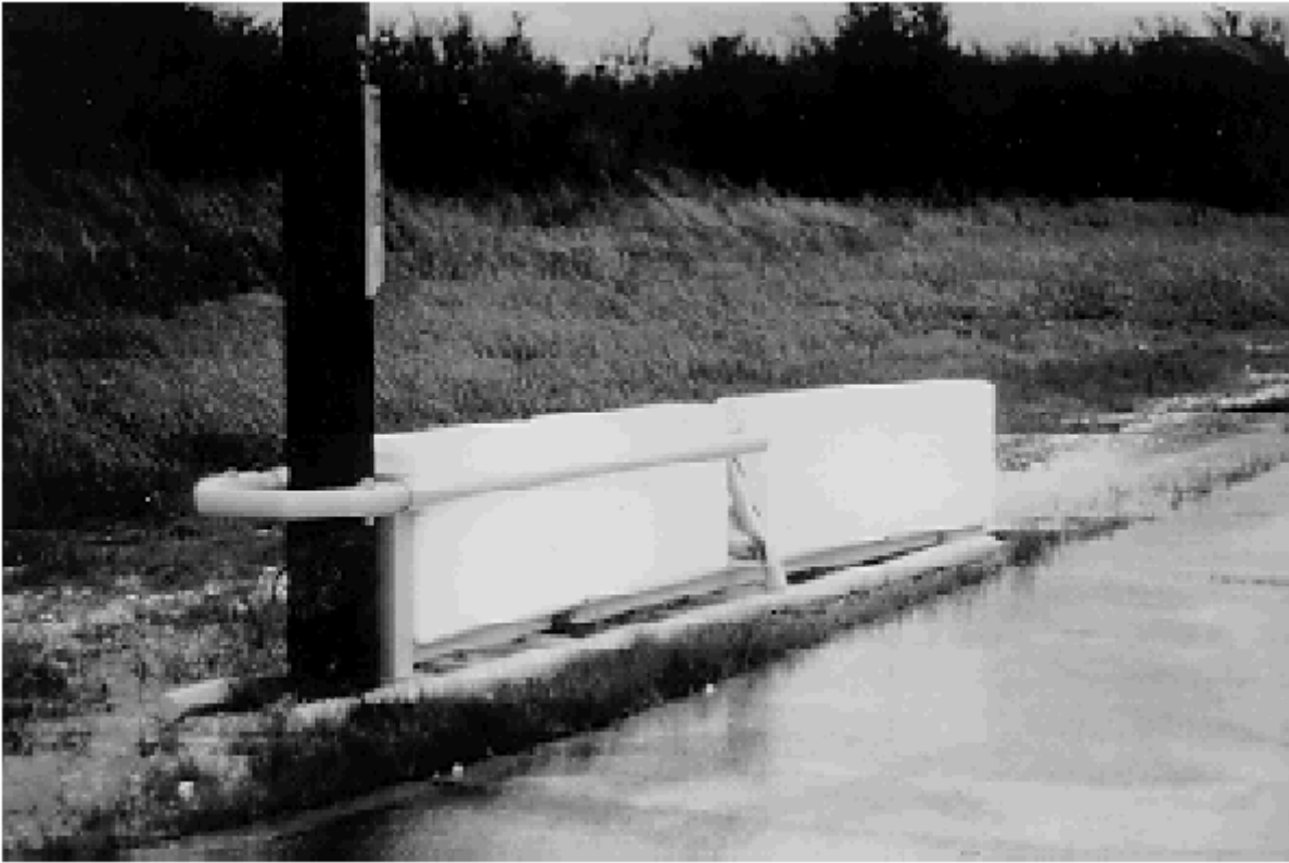
Figure 4a. ADIEM, Level 2 (soft concrete crash cushion)
