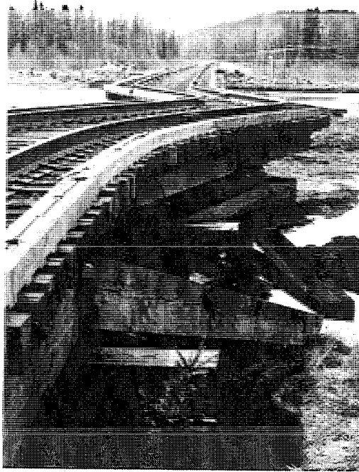
Figure 5. Stream bank convergence of about 0.18 m buckled the deck of the Alaska railway bridge at milepost 63.0 (after McCulloch and Bonilla (6)).
