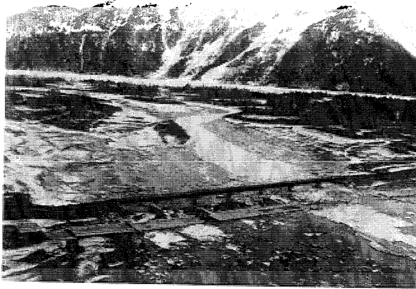
Figure 7. Collapsed highway bridge across Twentymile River (bridge nearest camera); damaged but intact railway bridge behind highway structure (after McCulloch and Bonilla (6)).
