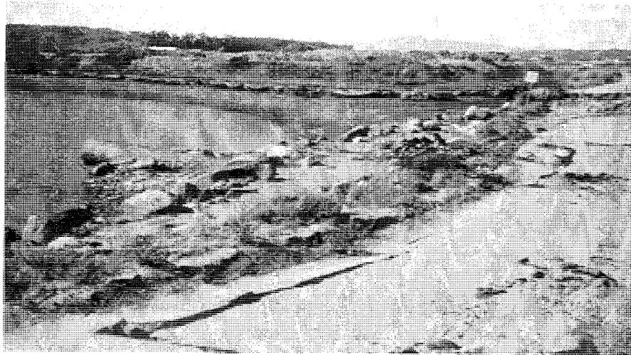
FIGURE 3 Damage to Jetty Road North of Moss Landing, California. View southeastward of Disturbed Embankment and Deflected End of CMP Culvert (Photograph by Ken Gray, Dept. of Parks and Recreation, Monterey County, Calif.)
