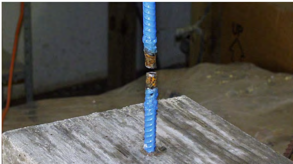
Figure 5.6: Typical Nylon Weld Fracture
