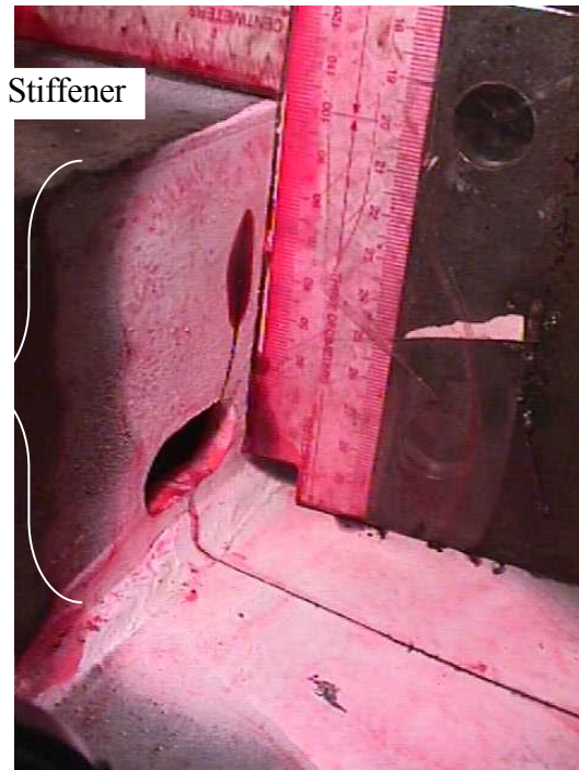
Figure 3-17: Crack growing in stiffener of case 3.
