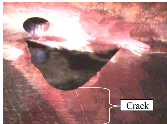
Figure 11-17: Detail of crack at prepared weld access hole prior to welding.
