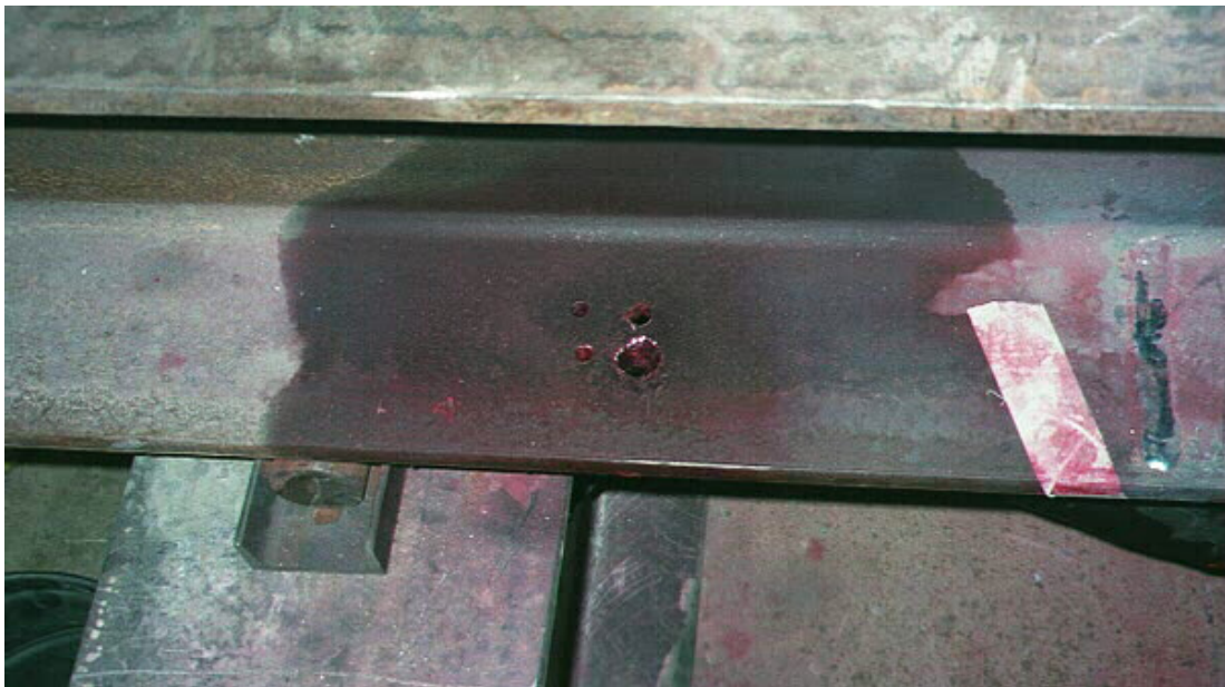
Figure 11-39: Several cracks arrested by hole drilling.
