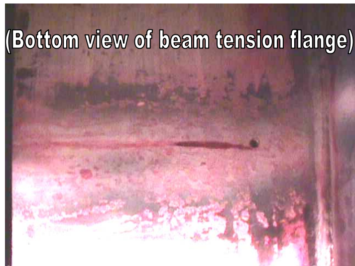
Figure 11-34: Initial hole drilled which missed the crack tip.
