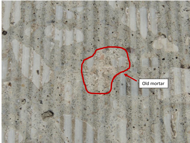
Figure 7. Identification of RCA with Old Mortar from the Field Survey in I-40 EB Segment 3.
