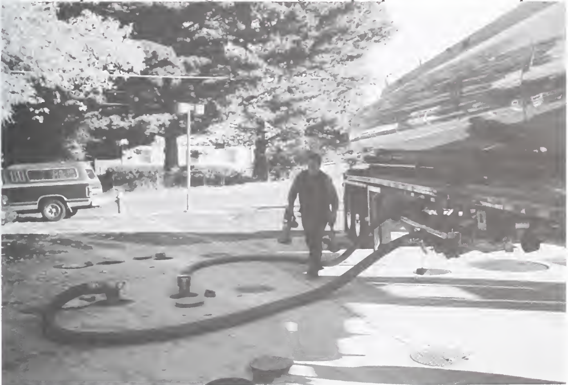
At gas station, driver unloads & emplaces connector fittings & hoses to underground tanks
