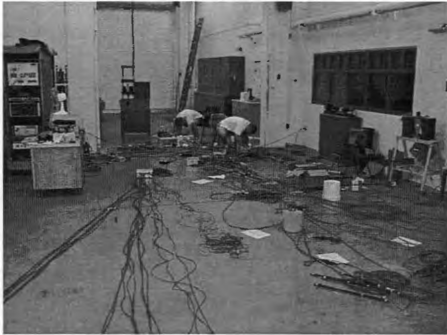
Figure 2.10 Instrumentation and associated wires being readied for placement in the girder molds at the precasting site
