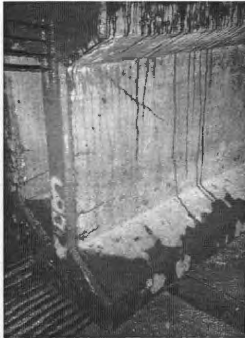
Figure 5.18 Photograph of girder end cracking
