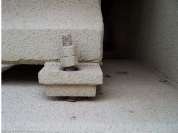
a) Bent anchor bolts on the eastern abutment bridge seat
