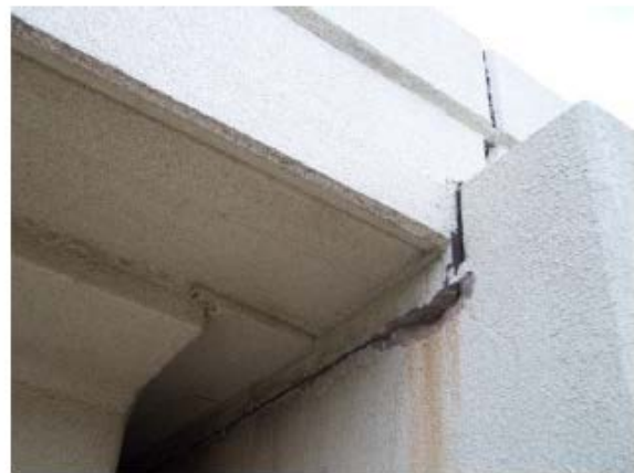
d) Large crack in the eastern abutment back wall
