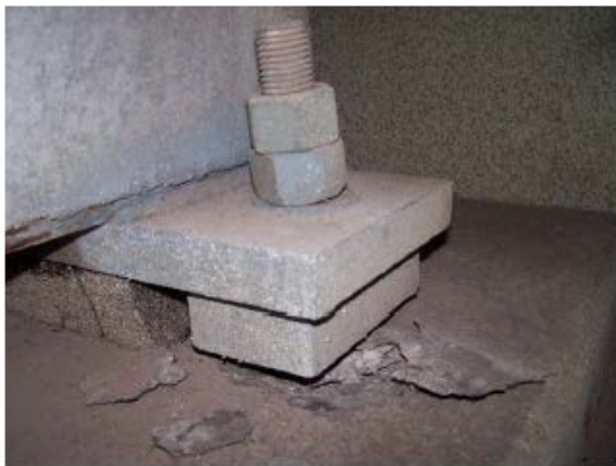
c) Bent anchor bolts with deformed elastomeric bearing pads on the eastern abutment bridge seat
