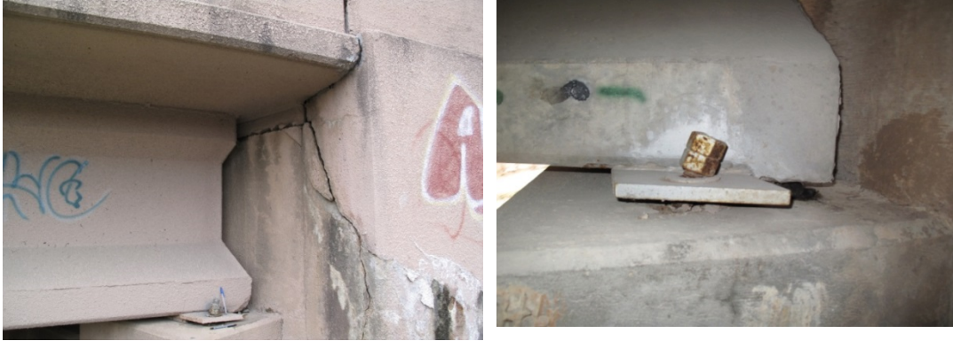
Figure 36. Beams pushing against abutment backwalls and a bent anchor bolt
