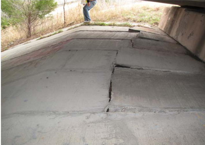
Figure 37. Cracks in the slope-wall
