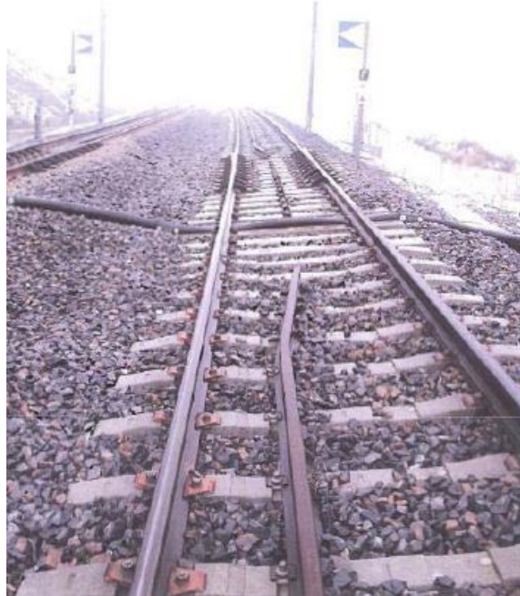
Figure 3.4 Guard rail protection (Abtahi, 2013)
