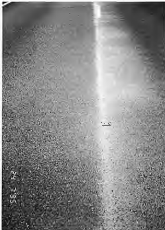
b) Staining at Joint, MP 134.5
