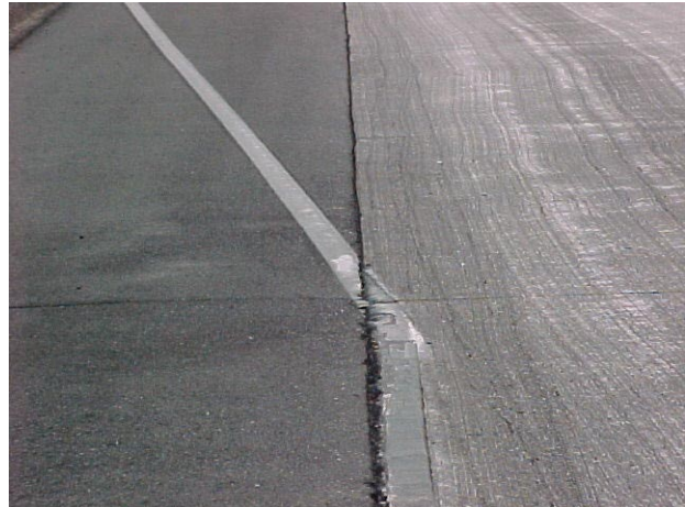
Fig. 11: Epoxy Taper Line in Back Ground Adjoining a White Lumimark Edge Line
