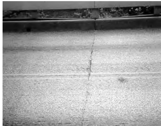
Figure 4.17 Cracked Slab over Floor Beam
