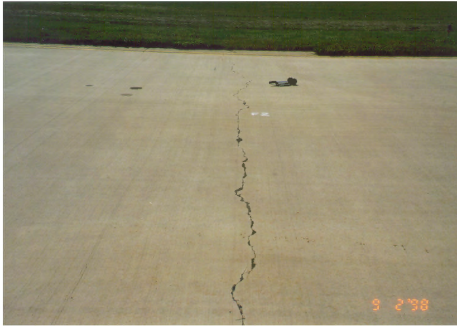
FIGURE B-17. CRACK NO. 2 IN THE FIBROUS PAVEMENT, A TRANSVERSE CRACK WHICH OCCURRED IN OCTOBER 1993 (SEPT. 1998)
