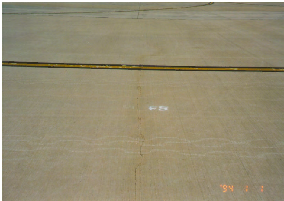
FIGURE B-18. CRACK NO. 5 IN THE FIBROUS PAVEMENT, A TRANSVERSE CRACK (SEPT. 1998)
