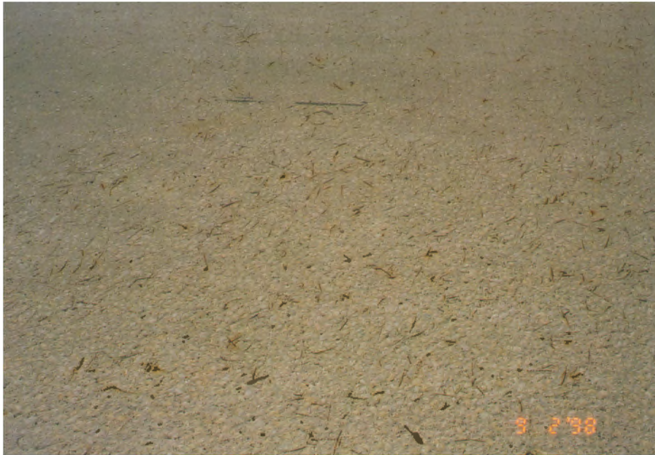
FIGURE B-3. LOSS OF MORTAR DUE TO CONSTRUCTION TRAFFIC (SEPT. 1998)
