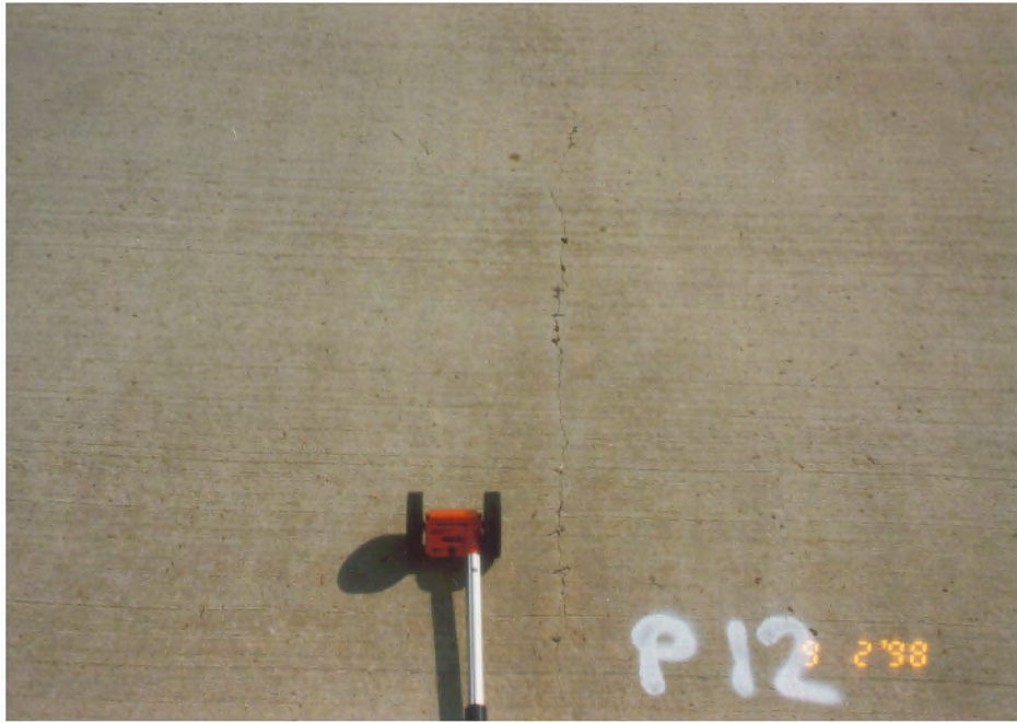
FIGURE B-13. CRACK NO. 12 IN THE PRESTRESSED PAVEMENT, A LONGITUDINAL CRACK (SEPT. 1998)
