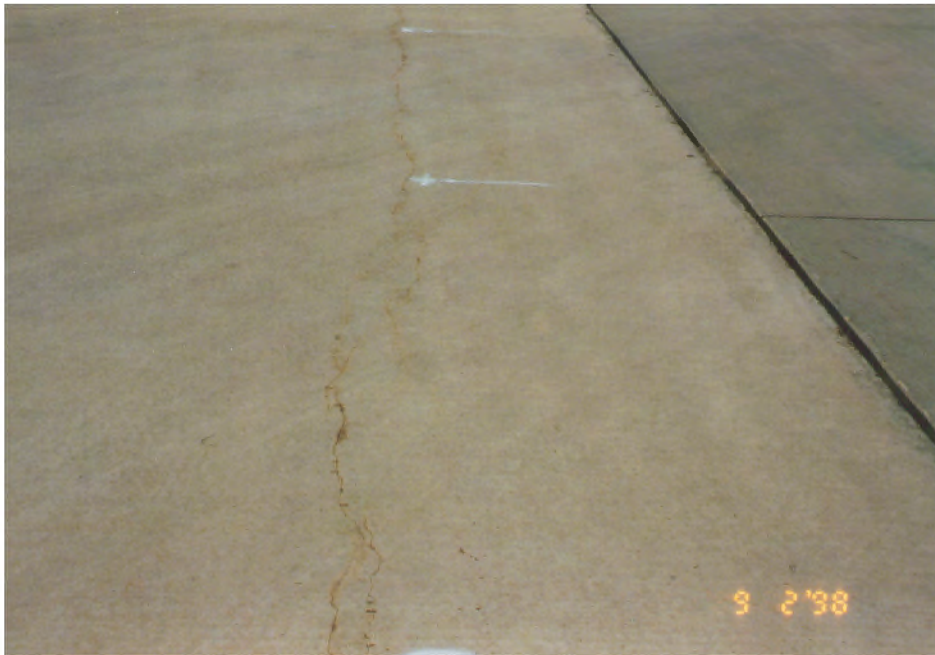
FIGURE B-16. LONGITUDINAL CRACK NO. 2 ALONG PAVEMENT EDGE (SEPT. 1998)
