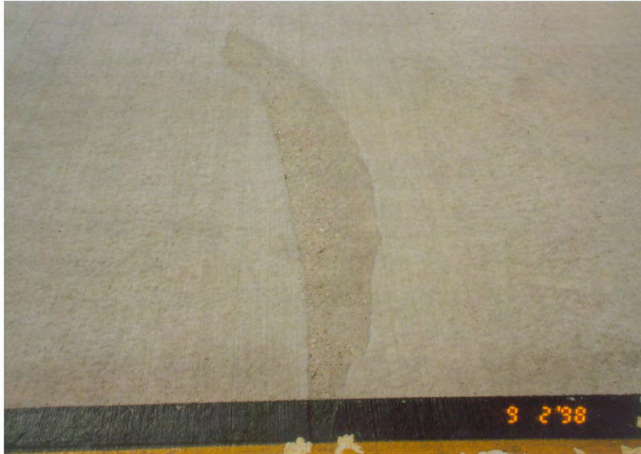
FIGURE B-4. SURFACE DAMAGED BY RAIN DURING CONSTRUCTION (SEPT. 1998)
