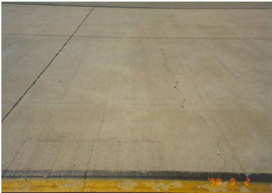
FIGURE B-26. TRANSVERSE CRACK IN CONVENTIONAL PAVEMENT (SEPT. 1998)
