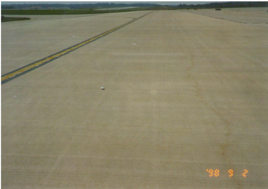
FIGURE B-24. LONGITUDINAL CRACK IN FIBROUS PAVEMENT, IN AIRCRAFT WHEEL PATH (SEPT. 1998)
