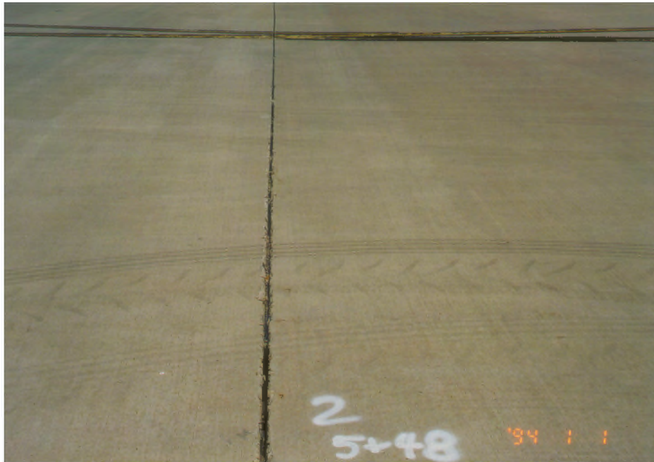
FIGURE B-21. JOINT, STA. 5+48 IN FIBROUS PAVEMENT, A WORKING JOINT (SEPT. 1998)
