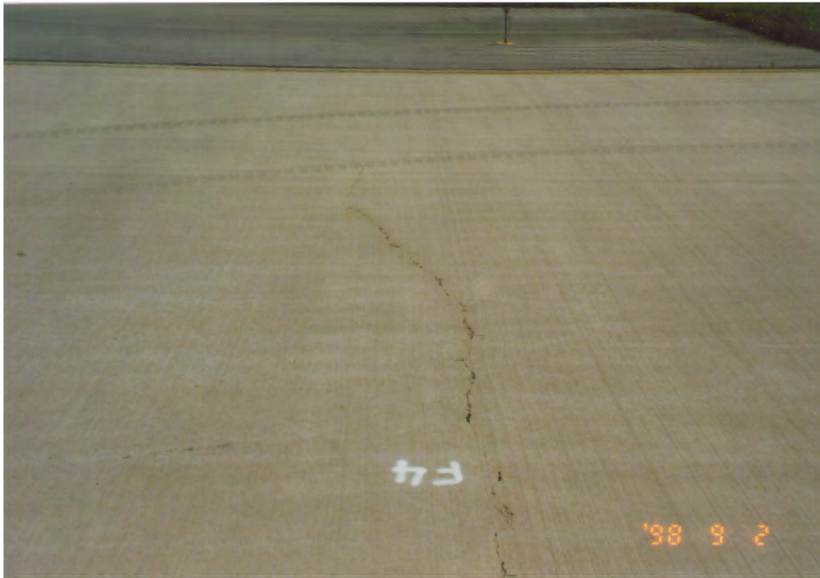
FIGURE B-19. CRACK NO. 4 IN THE FIBROUS PAVEMENT, A TRANSVERSE CRACK (SEPT. 1998)
