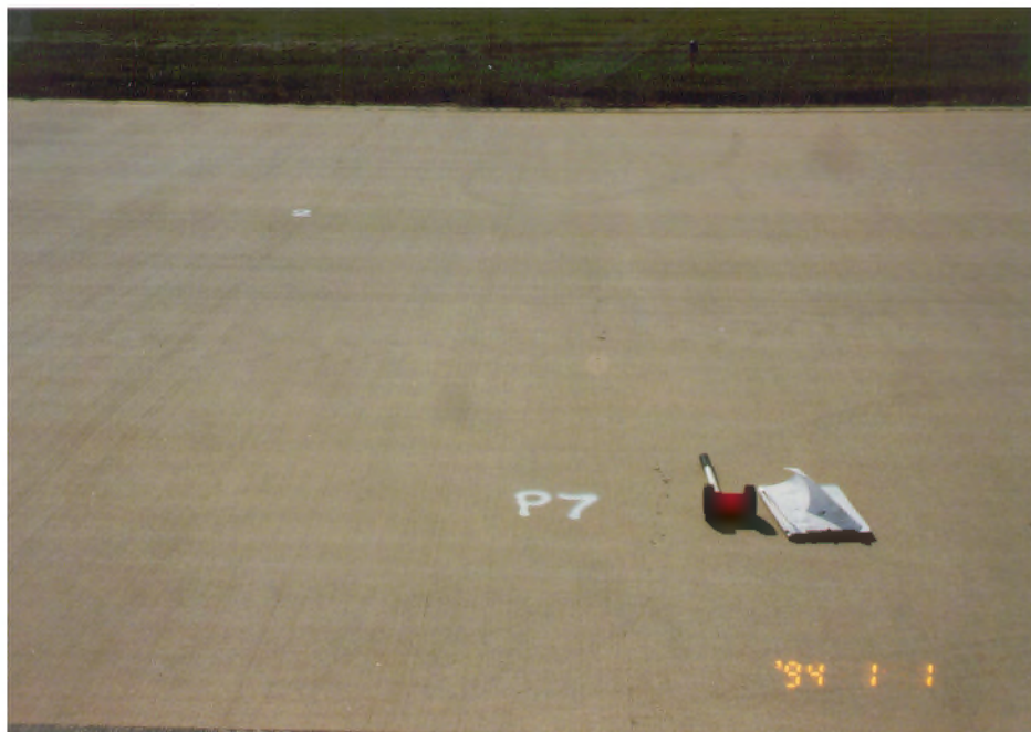
FIGURE B-12. CRACK NO. 7 IN PRESTRESSED PAVEMENT, A TRANSVERSE CRACK (SEPT. 1998)
