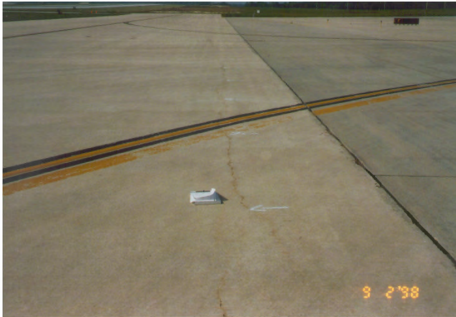
FIGURE B-15. LONGITUDINAL CRACK NO. 1 ALONG PAVEMENT EDGE (SEPT. 1998)
