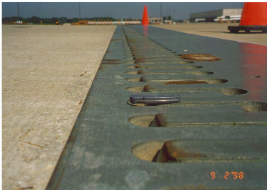
FIGURE B-8. CLOSE-UP OF THE FINGER JOINT, NOTE ELEVATION DIFFERENCE (SEPT. 1998)
