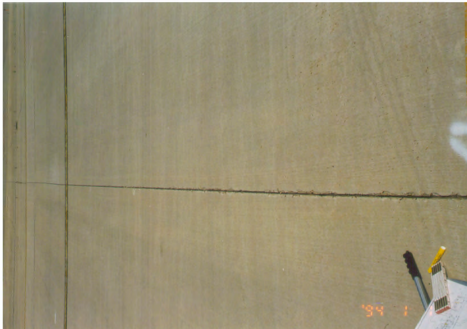
FIGURE B-22. JOINT, STA. 7+48 IN FIBROUS PAVEMENT, A WORKING JOINT (SEPT. 1998)
