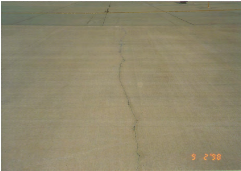
FIGURE B-9. PAVING CRACK NO. 1 IN PRESTRESSED PAVEMENT (SEPT. 1998)
