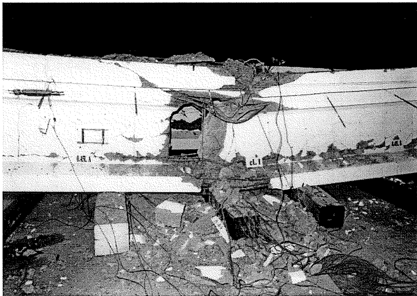
Figure 10.9 Heavily Damaged Region – Girder I
