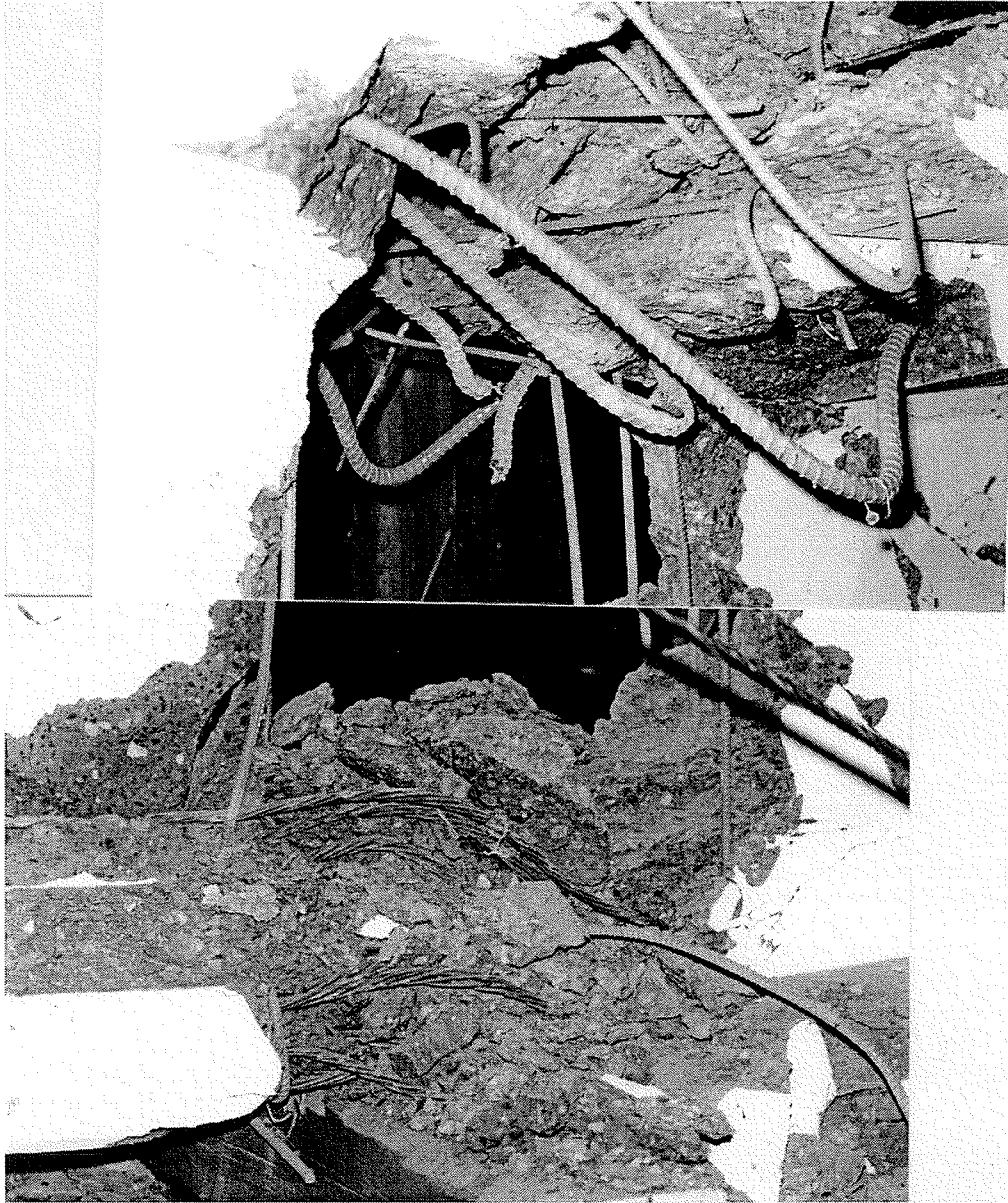
Figure 10.15 Close-up of Damaged Region – Girder II
