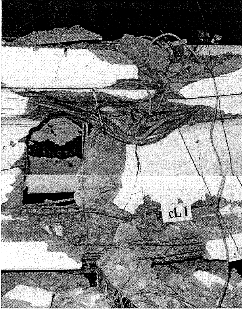
Figure 10.10 Close-up of Damaged Region – Girder I
