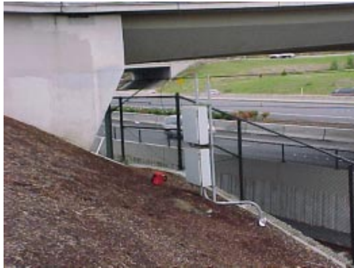
Figure 7.1: Wall 13 control panel
