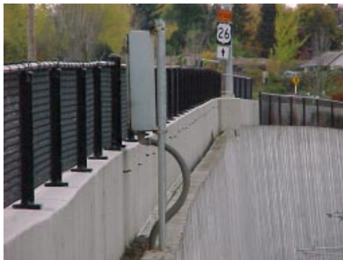
Figure 7.2: Wall 14 control panel
