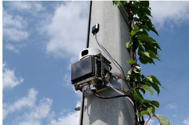
Figure 4-1 Radar (large black box) mounted on pole with covert camera (in white housing) and GPS antenna (small black box above radar)
