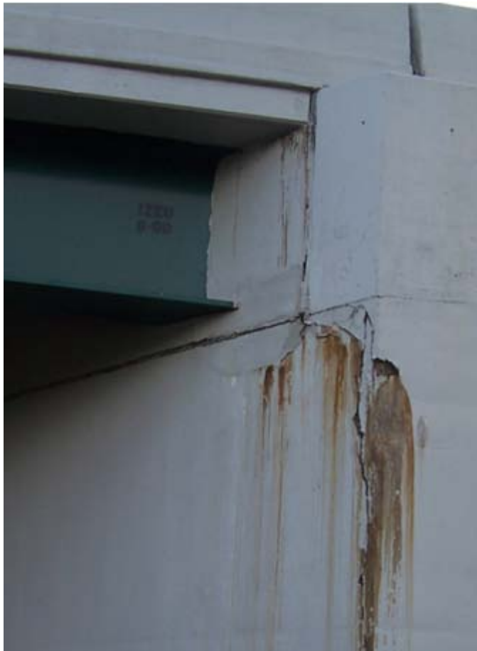
Figure 11: Observed Distress of West Wall (West Bound Bridge)
