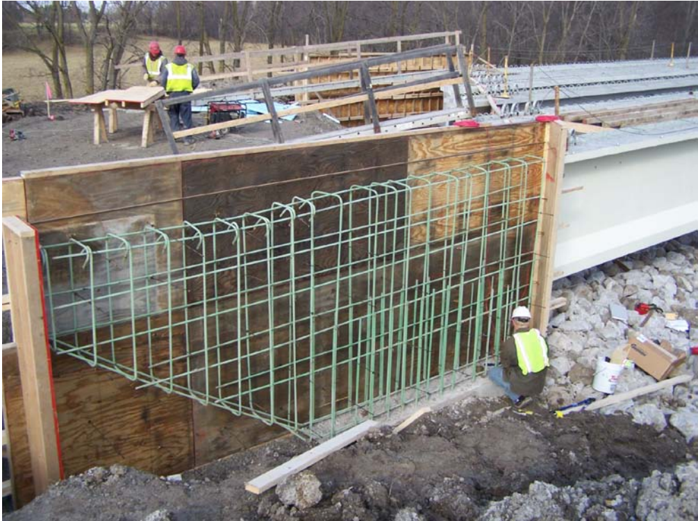
Figure 15: Vibrating Wire Strain Gage Installation
