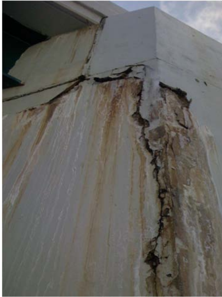
Figure 13: Propagated Cracks of West Wall (West Bound Bridge)
