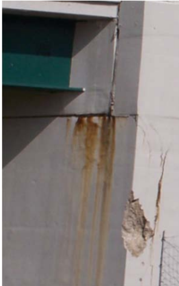
Figure 12: Observed Distress of East Wall (East Bound Bridge)
