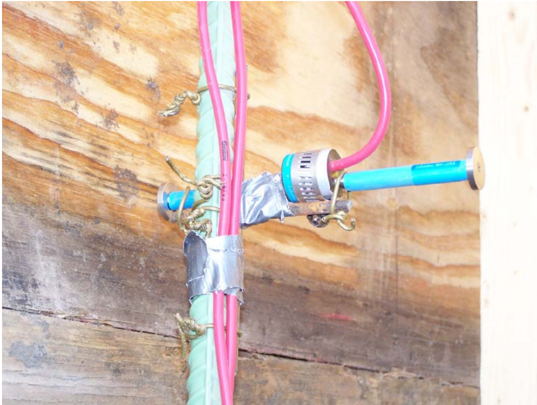
Figure 16: Vibrating Wire Strain Gage Tied to Reinforcement
