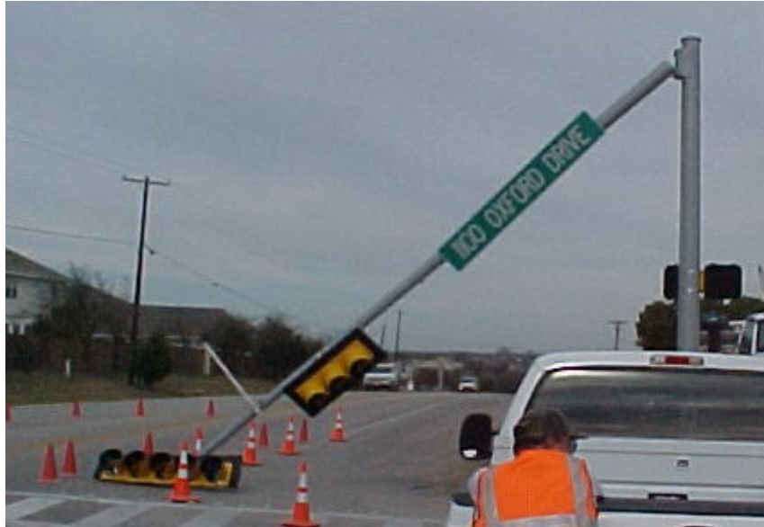
Figure 1.1: Falling Cantilevered Highway Sign Structure
