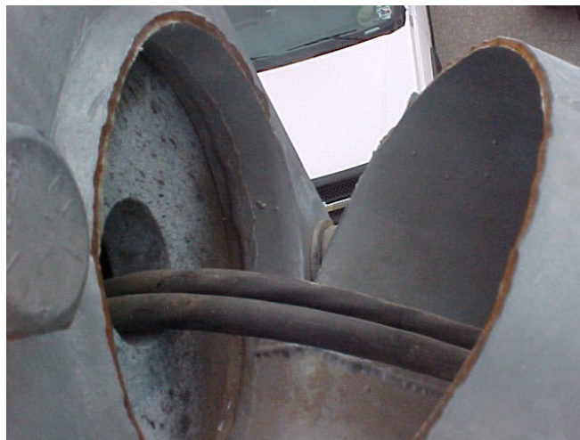
Figure 1.2: Fatigue Failure at Mast Arm Connection of Traffic Signal
