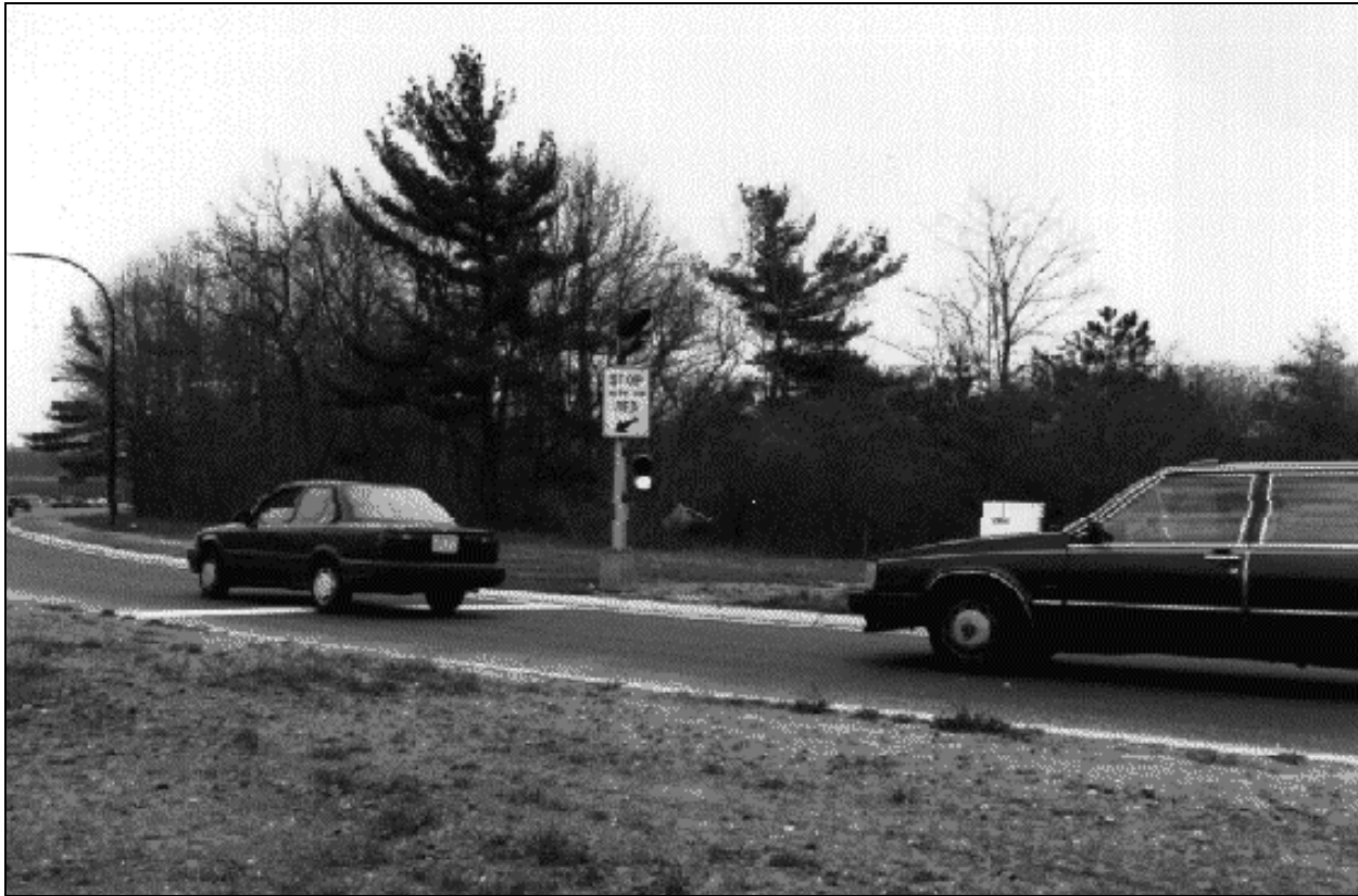
Figure 4-15. Ramp metering signals.
