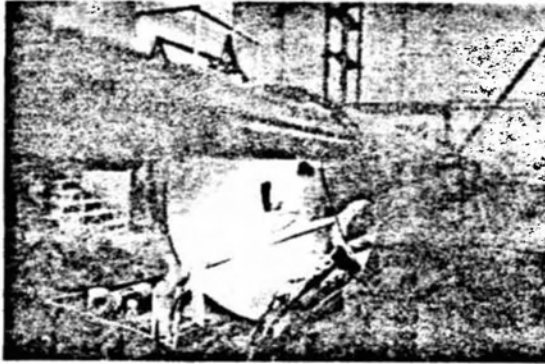
a. Ribbon cable wires ready for attachment to barrier terminal. LPC tubing and extensometer tube also visible
