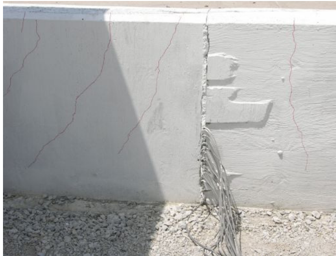
Figure 21. System Damage, Back Side Concrete Cracks, Test CBPP-1
