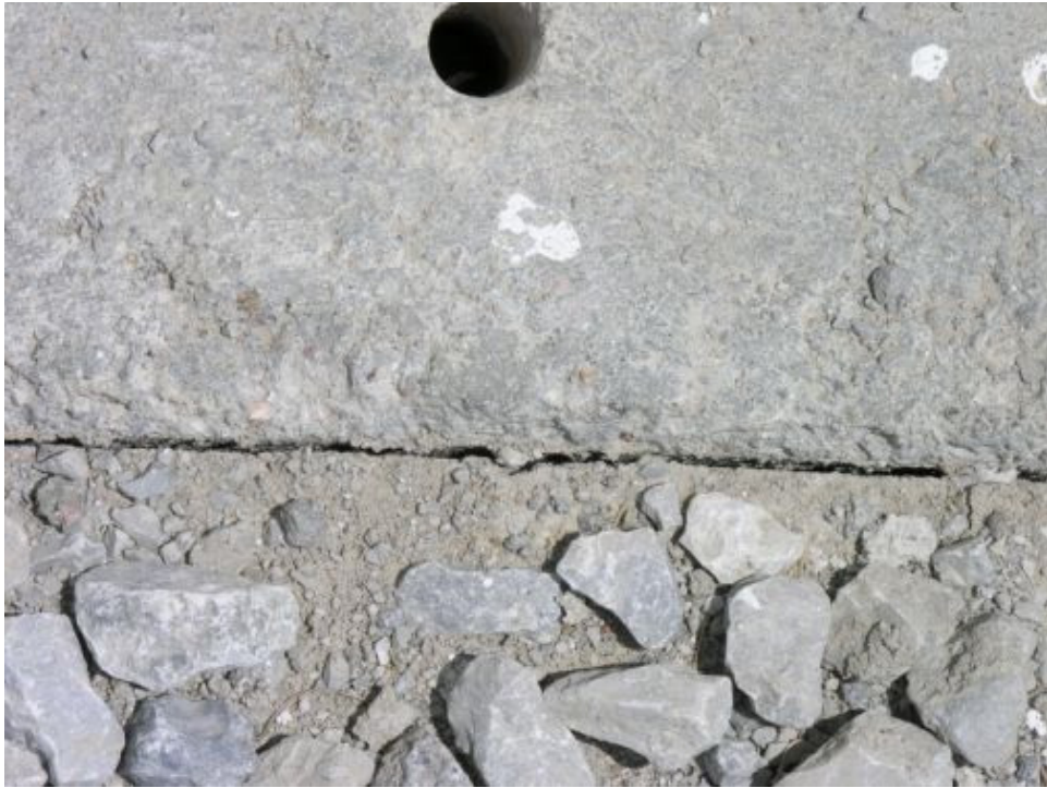
Figure 22. System Damage, Soil Gap, Test CBPP-1
