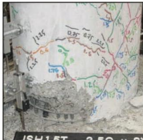
DS-5: imminent failure
