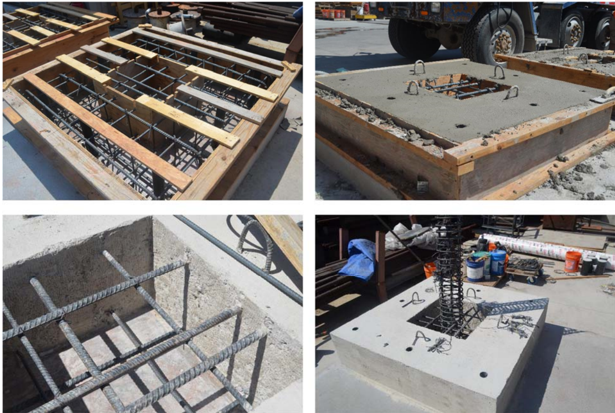
Figure 4-2 Casting of NSC footing and roughening of the inner surface of the footing.
