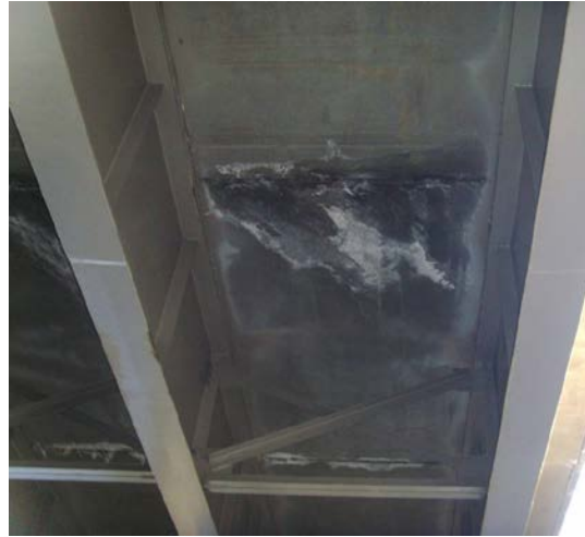
Figure 2.15: Typical joint leakage at deck panels (I-84 WB over Weber Canyon with welded-tie connections from 2009 inspection)[8]
