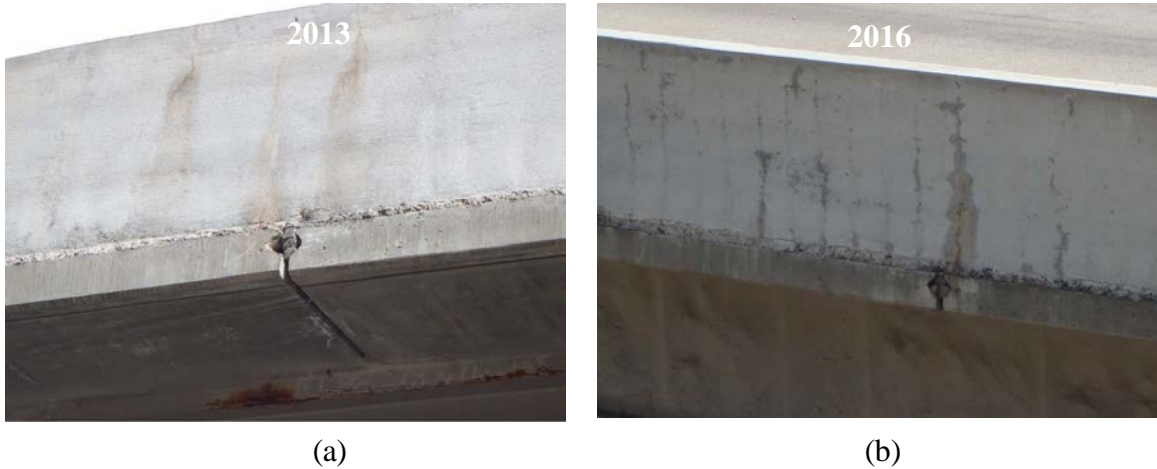
Figure 2.17 Cracks with efflorescence in parapet over the deck panel joint and Poorly bonded grout in shear pocket, I-84; US-89 to SR-167, Weber Canyon (Built 2008), Joint connection: Welded Tie connections [12]
