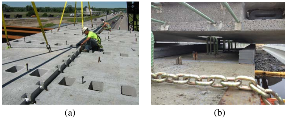
Figure 2.3: Common shear pockets used to create composite action between beams and deck; shear studs grouped improve constructability used in (a) 24 th Street Bridge over I-29/I-80 (Iowa, 2008) and (b) TH 53 Bridge over Paleface River (Minnesota, 2012) [5]
