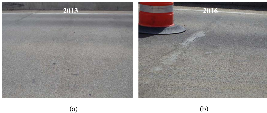
Figure 2.16 Typical transverse cracking in the overlay which worsened from 2013 to 2016, I-84; US-89 to SR-167, Weber Canyon (Built 2008)-Joint connection: Welded Tie connections [12]
