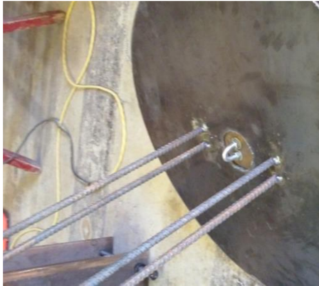
Figure 40. CMP lid with reinforcing bar guides and U-bolt
