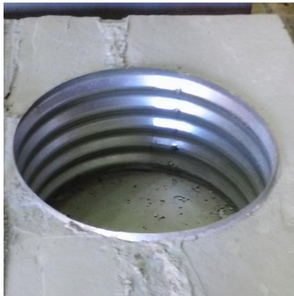
Figure 39. CMP void in pile cap
