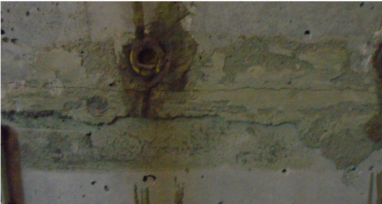
Figure 72. Crack between grout bed and diaphragm
