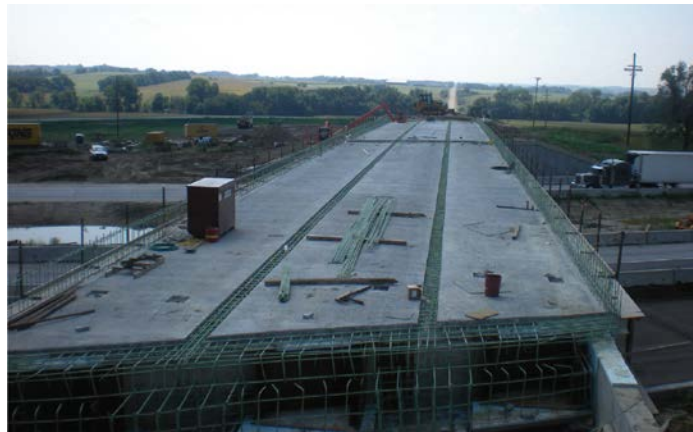
Figure 10-4 Completing the placement of the pre-topped units for the bridge over I-80 at 262nd Street in Nebraska (AZIZINAMINI, 2014).
