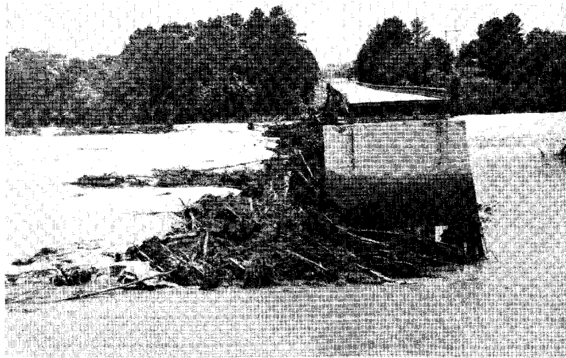
Figure 119. Damaged U. S. Highway Bridge over the Homochitto River at Rosetta, Mississippi after spring 1974 flood.
