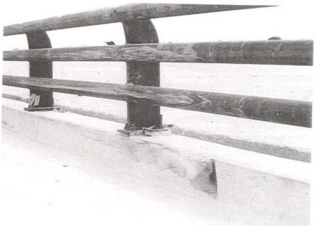
Figure 50. Bridge Rail Damage, Test GWMP-1.
