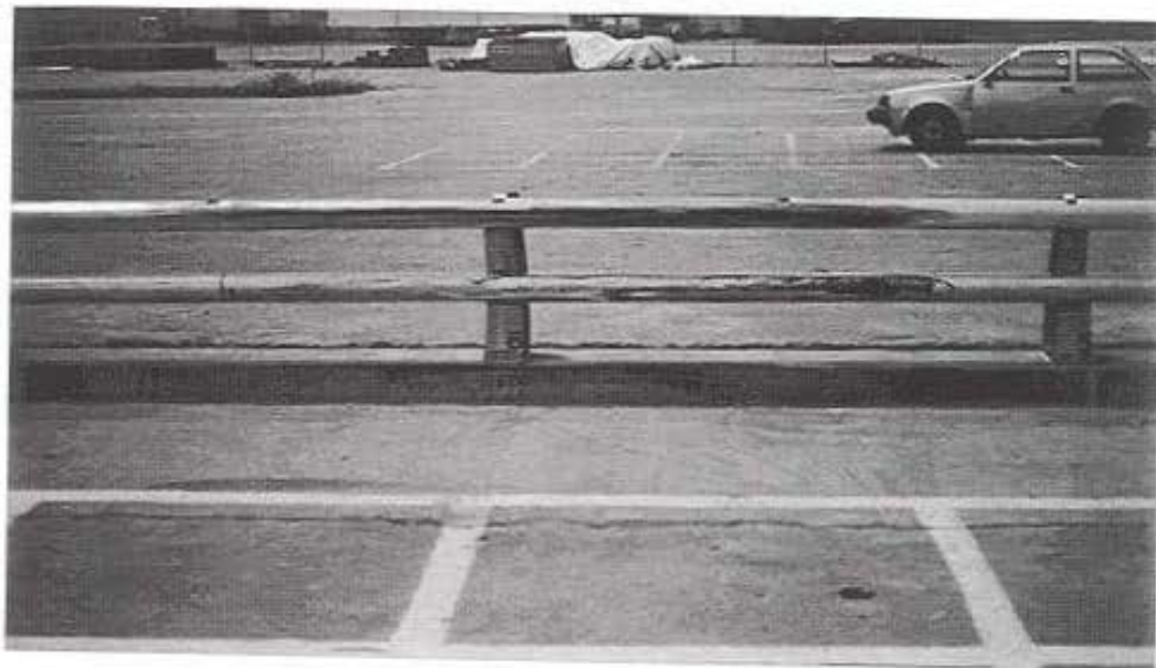
Figure 85. Bridge Rail Damage, Test FPAR-3.
