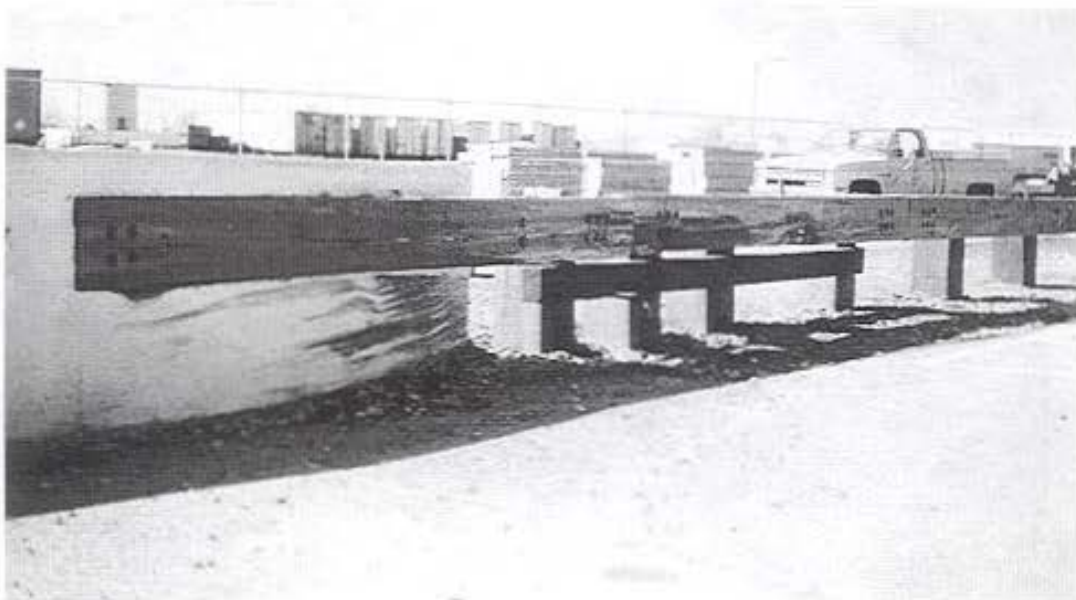
Figure 41. System Damage, Test SBT-5.
