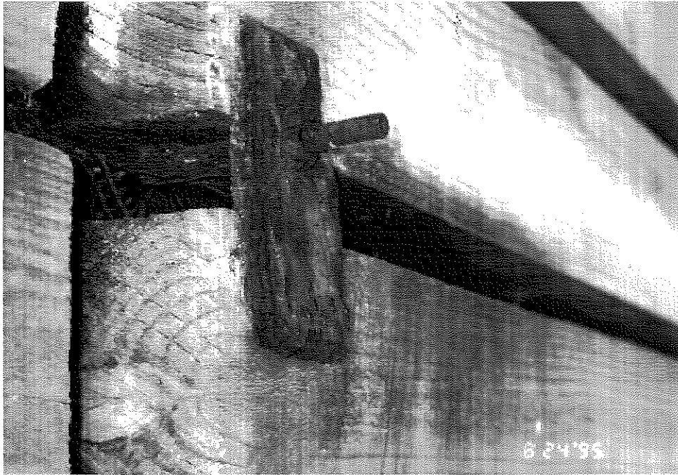
Figure 71: Rusted Timber Lagging Ties (Campbell County, US 27)
