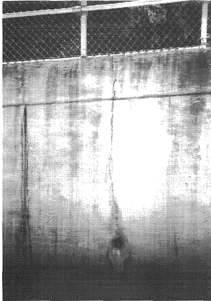
Figure 48: Cracking and Staining Stemming from Weep Hole (Floyd County)
