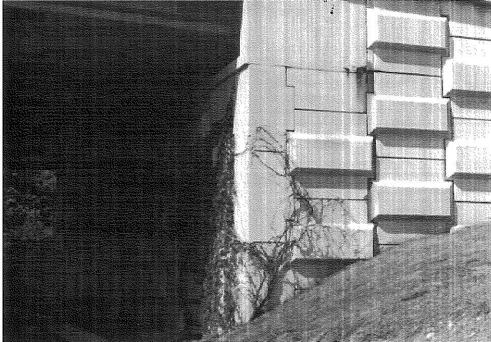
Figure 98: Staining & Vegetation Growing between Precast Panels (Fayette County, Jefferson St.)
