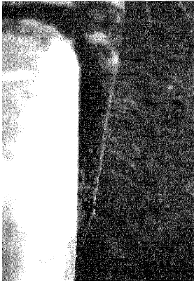
Figure 84: Forward Displacement of Precast Panel (Boone County, I-75 S.B. & Mall Rd.)
