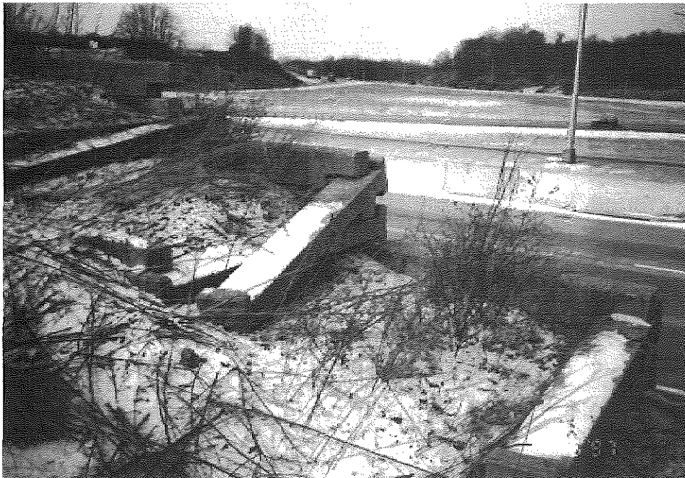
Figure 11: Sluffing of Unanchored Ends. (I-75 & I-75 Interchange)
