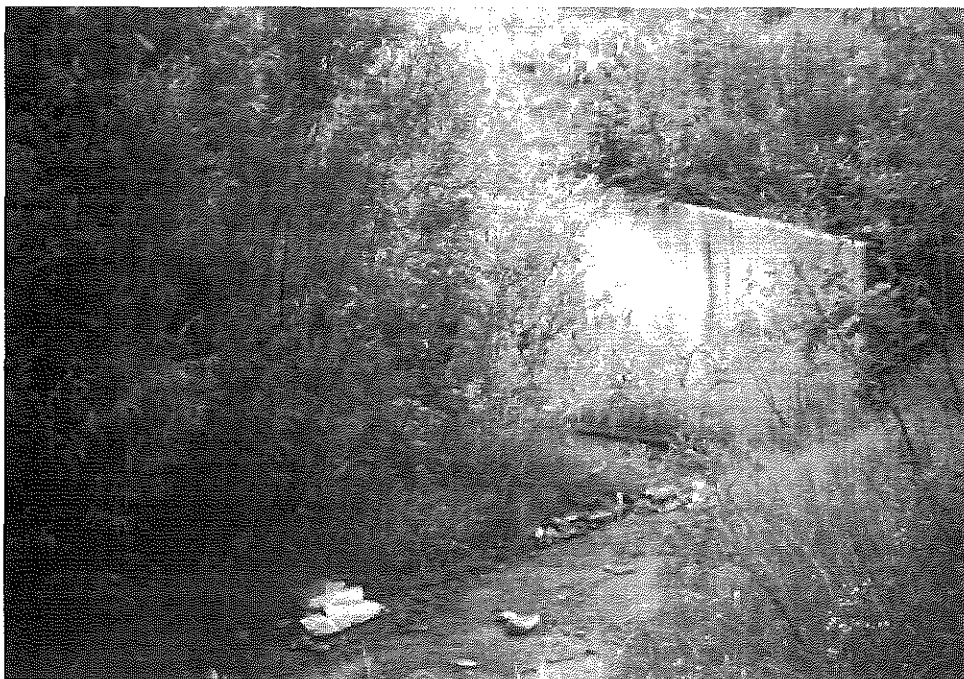
Figure 27: Vegetation in Culvert Outlet (Bracken County, KY 9, Milepost 4.46)
