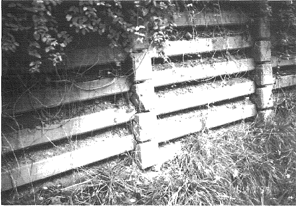
Figure 6: Migration of Backfill Through Open Face Crib Wall. (Lee County, US 52)
