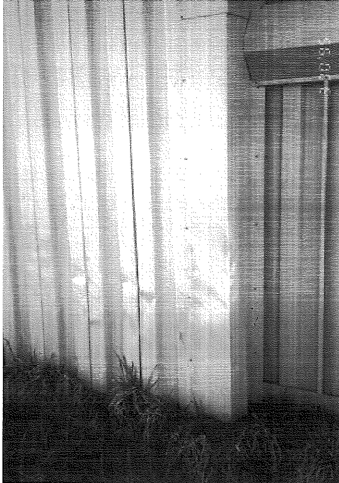
Figure 107: Dented Metal on Sound Wall Caused by Mowers (Scott County)
