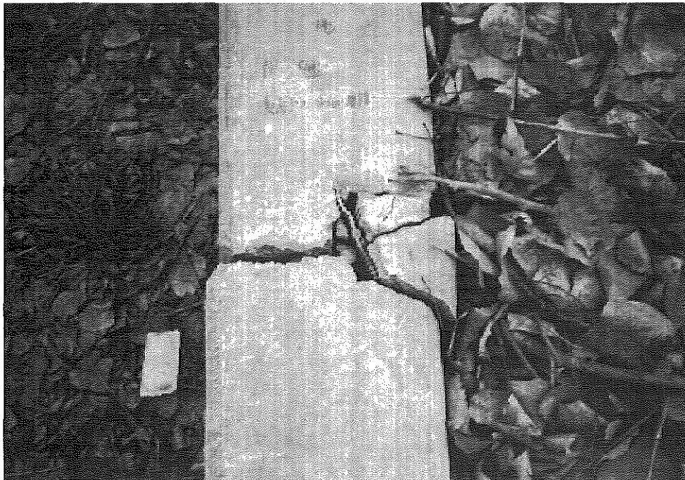
Figure 49: Sheared Key-Joint (Jefferson County, KY 1065)
