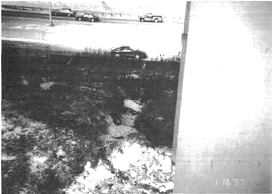
Figure 14: Erosional Channel Leading from Bridge Deck Drain to the Top of the Concrete Crib Wall. (I-71 & I-75 Interchange)
