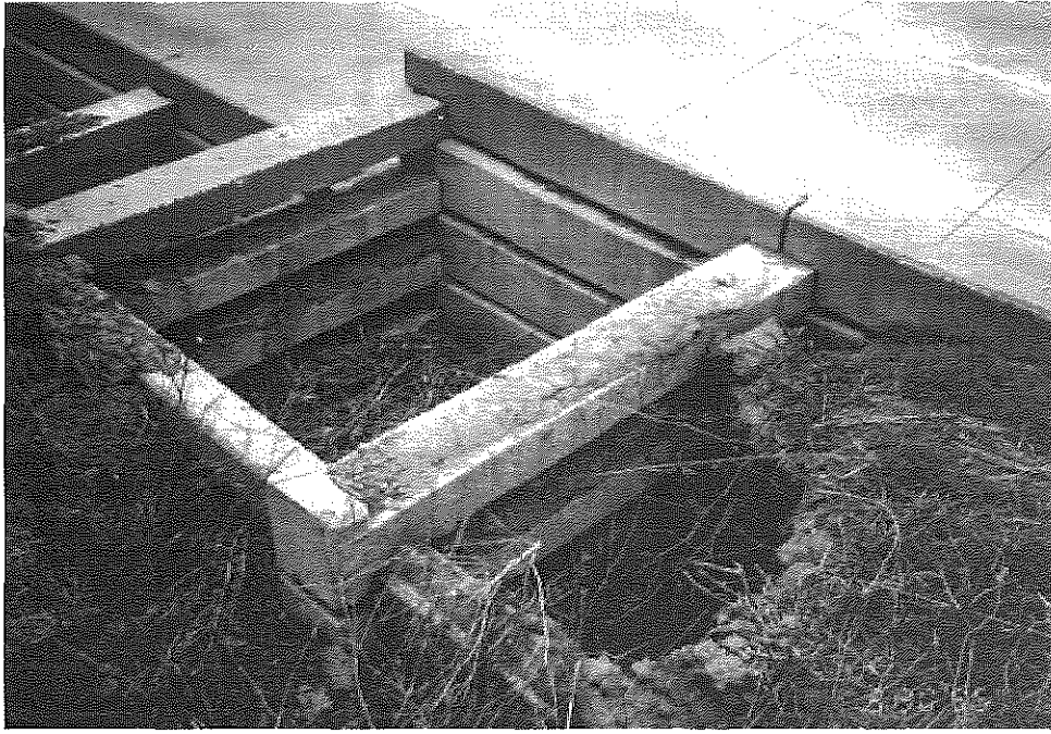
Figure 4: Settlement in Backfill between Crib Members. (I-75 and I-71 Interchange)
