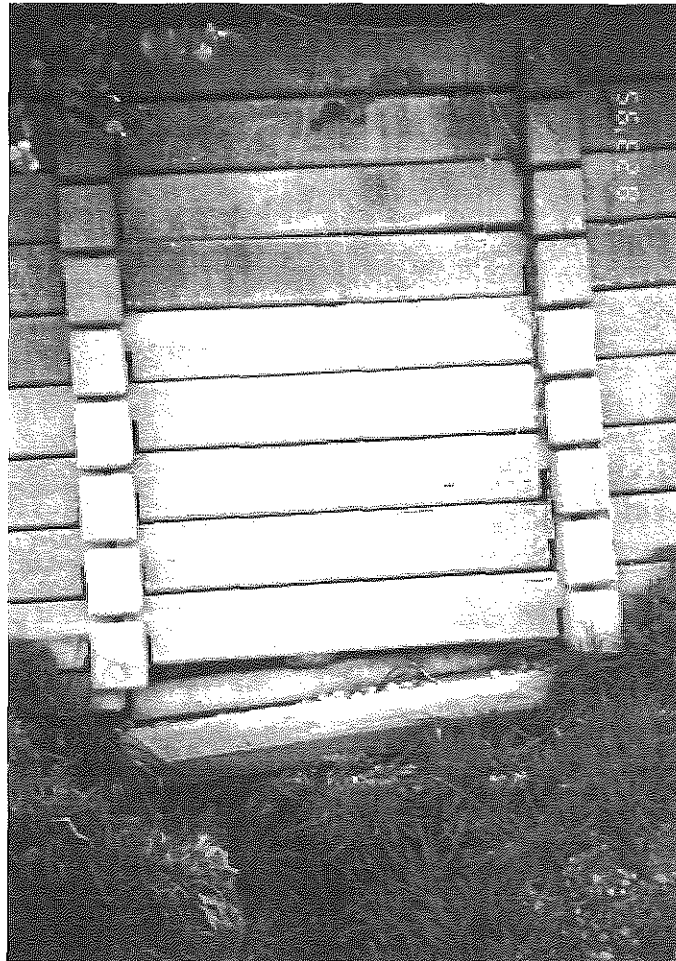
Figure 7: Displaced Crib Member Due to Erosion. (Kenton County, KY 8)
