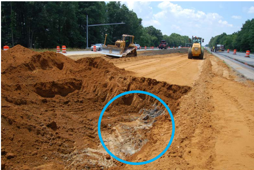
Figure 9. Undercutting of Section 2 revealing an underlying clay material.
