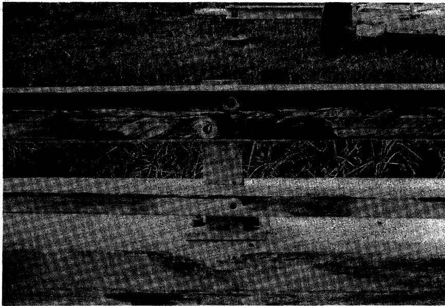
Figure 37. Damage at posts 5 and 6.
