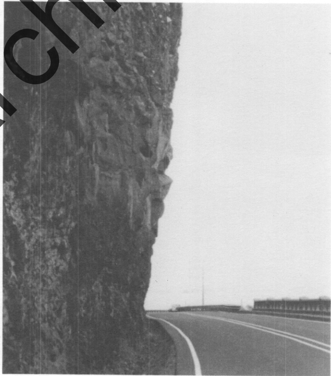
Figure 5.6 Rockfall from this slope will land on the roadway. No catchment is provided by the ditch.
