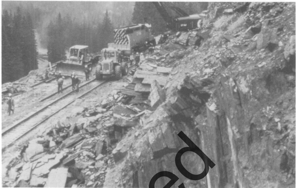
Figure 5.16 Note the toppling failures. This, too, is an adverse joint condition.
