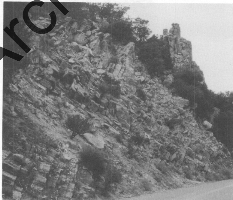
Figure 5.3 Determine the vertical height of the slope not the slope length. This 73-foot high slope is scored 25 points.
