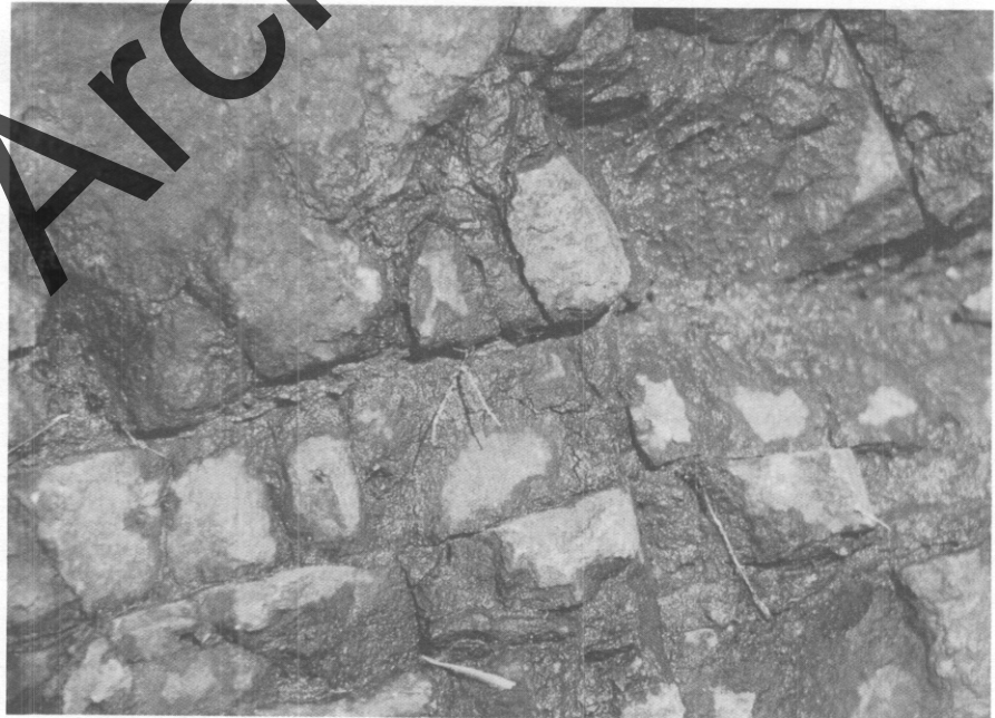
Figure 5.21 Weathered joint surface. Note the red colored clay between the rock surfaces.
