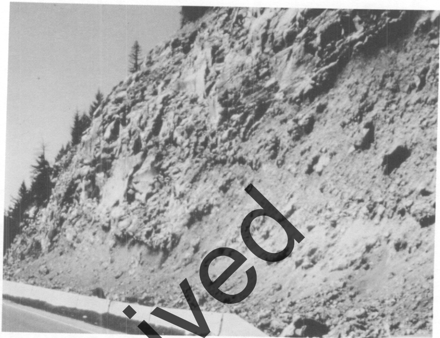
Figure 5.27 The cinders at the base of the slope are strongly affected by freeze/thaw cycles and rain. The difference is extreme.
