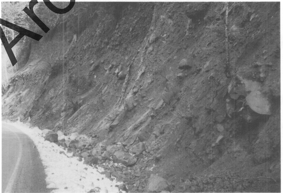
Figure 5.25 Oversteepened soil/rock slope
