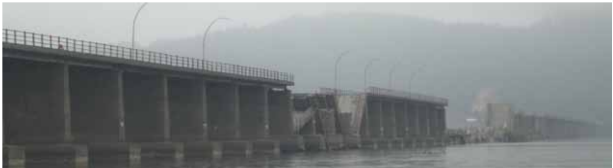
Figure 135. Photo. Collapsed spans in Biobío River bridge.
