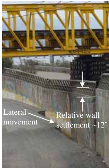
Figure 178. Photo. Settlement behind retaining wall on Chepe railroad bridge.
