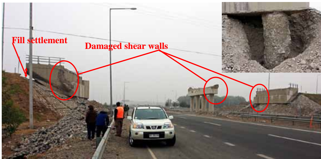
Figure 185. Photo. Damage at Romero bridge and shaft foundation supporting abutment (collapsed superstructure removed).
