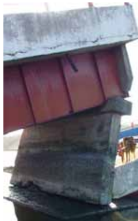
Figure 120. Photo. Tilting wall pier on Tubul bridge.
