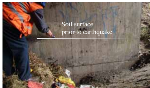
Figure 65. Photo. Soil surface on far side of undamaged column under approach to Juan Pablo II bridge.
