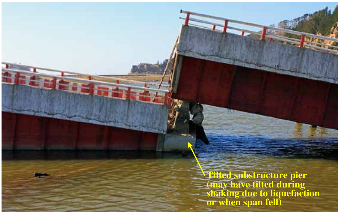
Figure 235. Photo. Collapsed and shifted spans at Raqui 2 bridge due to liquefaction.
