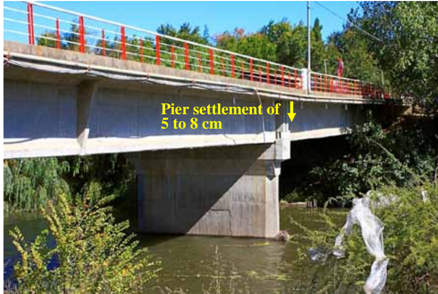
Figure 199. Photo. San Nicolás bridge center pier settlement probably due to liquefaction of soil layers beneath river.
