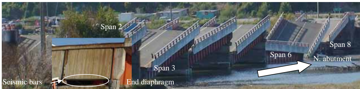
Figure 114. Photo. Unseating at southern ends of each span of Tubul bridge.
