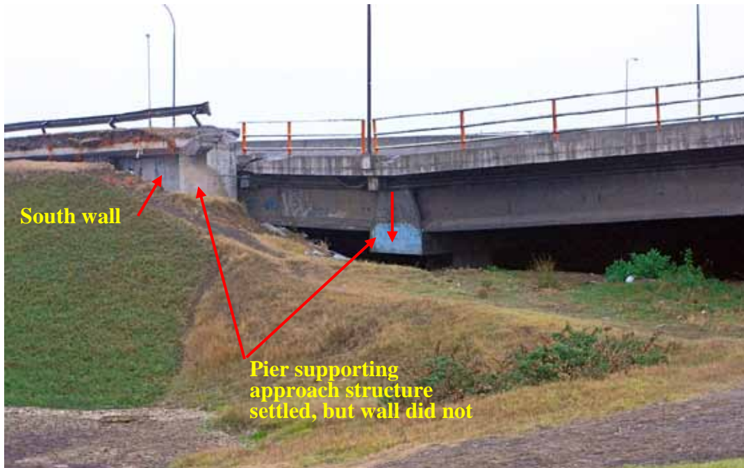
Figure 217. Photo. Settlement of approach structure for Juan Pablo II bridge.
