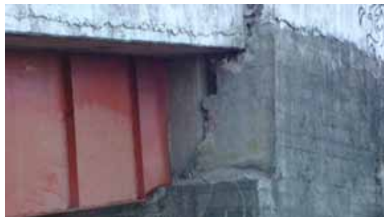
Figure 115. Photo. Punching of Tubul bridge deck into back wall
