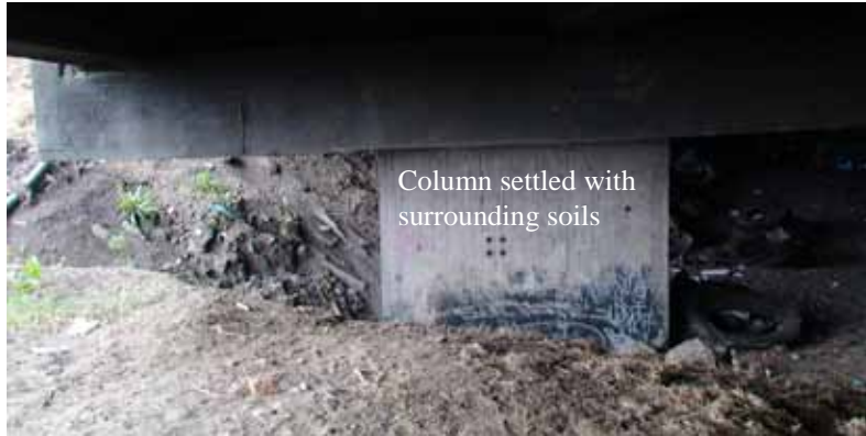
Figure 63. Photo. Column settlement under approach to Juan Pablo II bridge (cracks on far side).
