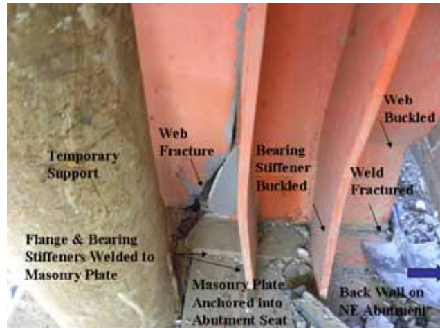
Figure 127. Photo. Girder damage at northeast abutment of Cardenal Raúl Silva Henríquez bridge.
