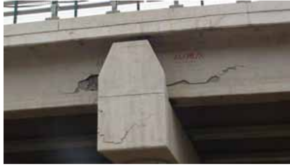
Figure 38. Photo. Curtain wall damage at bent of Chada bridge.
