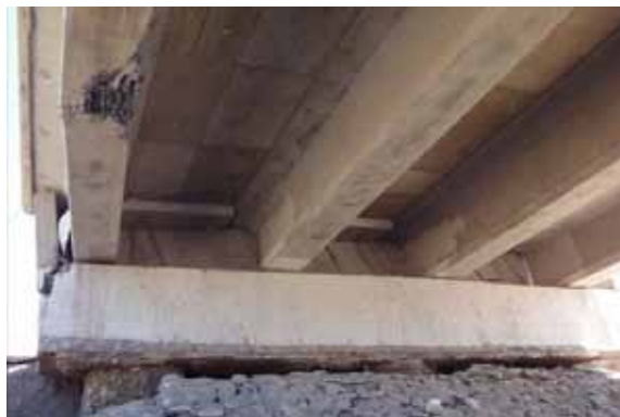
Figure 37. Photo. Bottom flange damage to Chada bridge.
