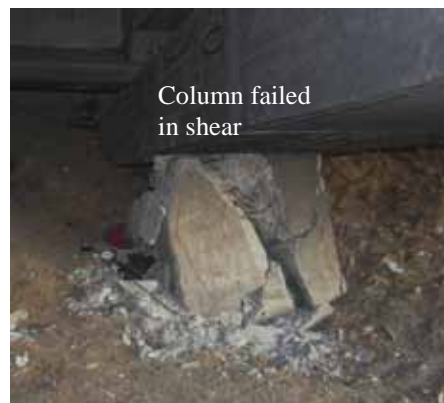
Figure 64. Photo. Reduced column height due to shear failure under approach to Juan Pablo II bridge.
