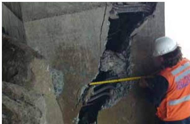
Figure 70. Photo. Back face of failure plane at northern end of Juan Pablo II bridge.
