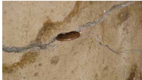
Figure 47. Photo. Close-up view of cracks at the level of rip rap on eastern approach to Llacolen bridge.
