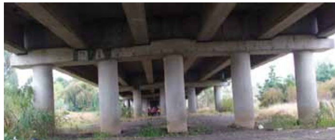
Figure 54. Photo. Columns with soil marks indicating ground settlement at west end of Llacolen bridge.
