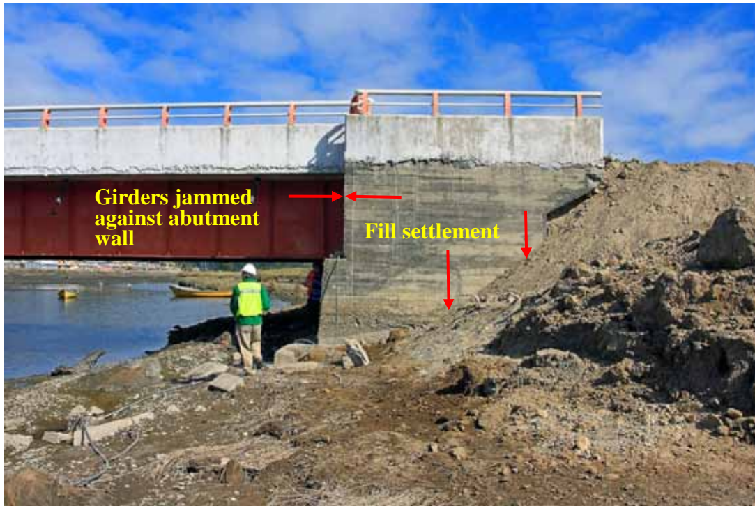
Figure 205. Photo. Abutment fill settlement at northwest abutment of Raqui 1 bridge.
