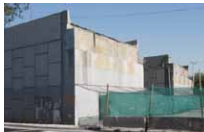
Figure 246. Photo. Retaining wall at Américo Vespucio/Miraflores.
