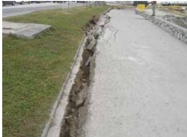
Figure 137. Photo. Lateral spreading near east end of Biobío River bridge.
