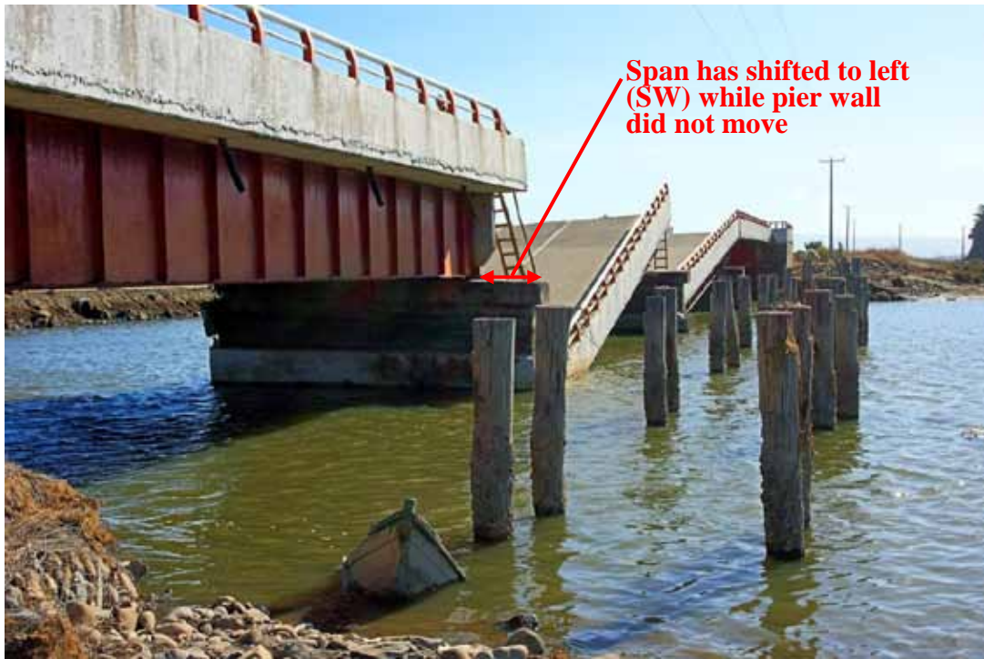
Figure 234. Photo. Collapsed and shifted spans at Raqui 2 bridge as viewed from base of southeast abutment.
