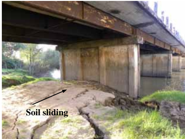
Figure 82. Photo. Sliding at south abutment under west Ramadillas bridge.
