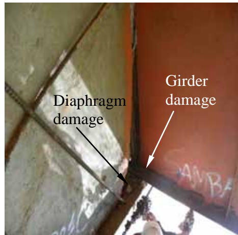
Figure 146. Photo. Diaphragm crushing in south abutment of Pichibudis bridge.
