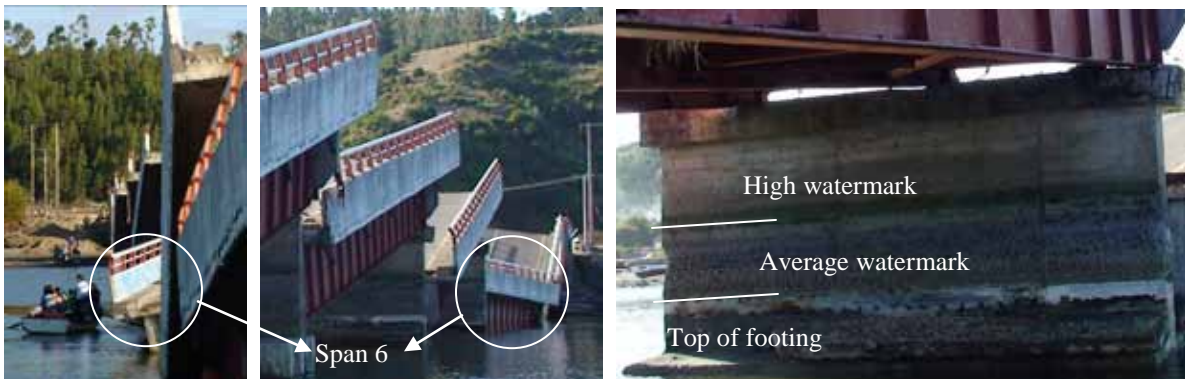
Figure 117. Photo. Span 6 of Tubul bridge, unseated at north end during an aftershock.
