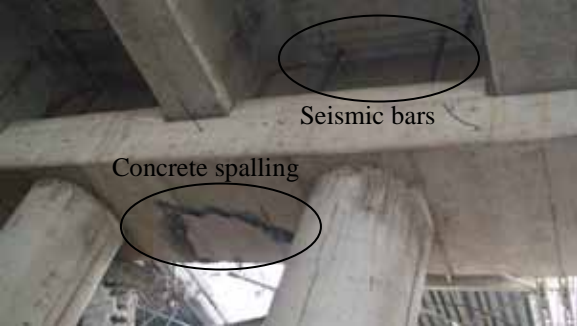
Figure 45. Photo. Concrete spalling beneath cap beam of eastern approach to Llacolen bridge.
