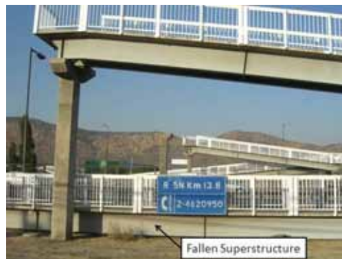
Figure 160. Photo. Damaged Route 5 pedestrian bridge.
