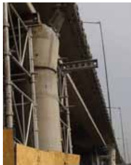
Figure 23. Photo. Damage to eastbound Independencia bridge.
