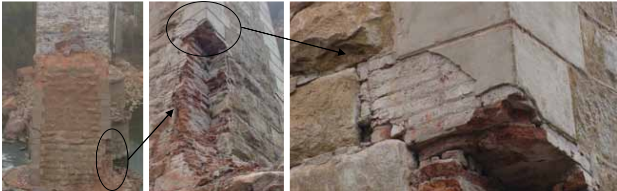
Figure 168. Photo. Pier of Claro River bridge.
