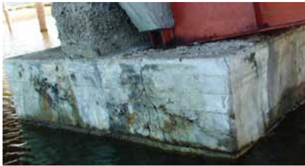
Figure 122. Photo. Crack in footing of Tubul bridge.
