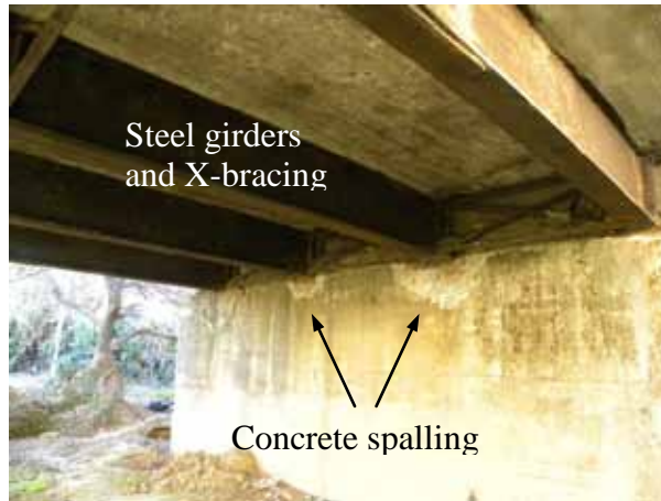
Figure 78. Photo. Abutment damage beneath west Ramadillas bridge.
