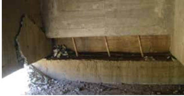
Figure 282. Photo. Exterior girder damage at San Nicolás bridge, partial diaphragms.
