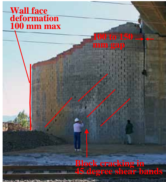
Figure 276. Photo. Wall with cracked block pattern at Muros Talca.
