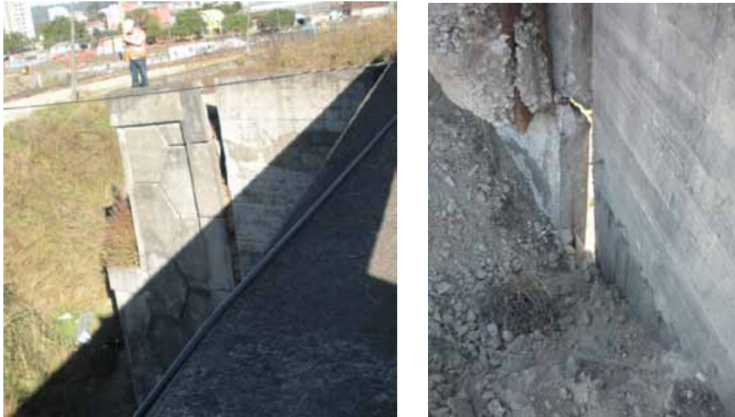
Figure 267. Photo. Tiered wall corner tilting outward at wall site 28A.
