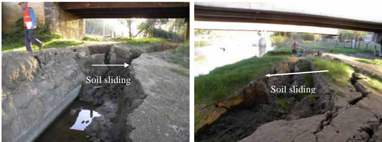
Figure 83. Photo. Block flow toward river due to liquefaction on south bank of Ramadillas bridges.
