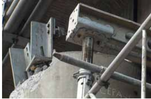
Figure 25. Photo. Damage to steel stoppers on eastbound Independencia bridge.
