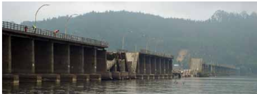
Figure 223. Photo. View of collapsed spans from northeast river bank of Biobío River.
