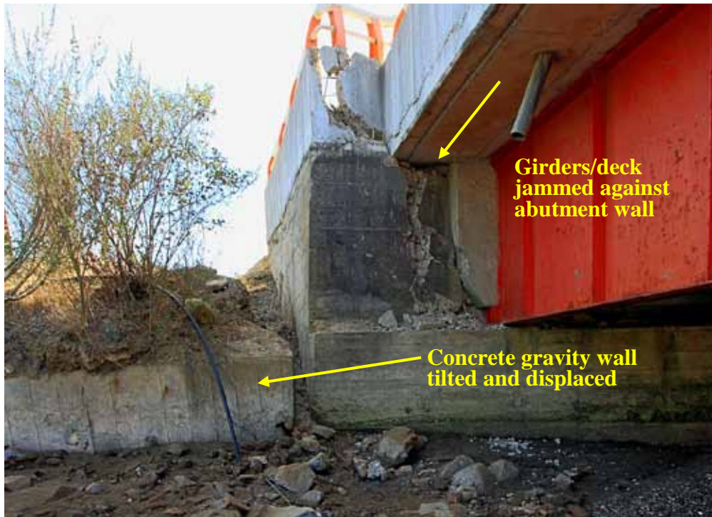
Figure 206. Photo. Abutment and girders shoved into each other and deck at the northwest abutment of the Raqui 1 bridge.
