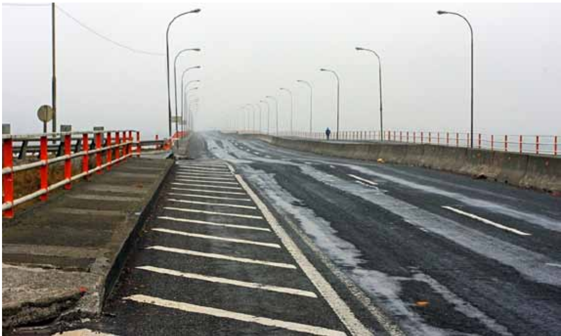
Figure 220. Photo. Roadway settlement due to settlement of mainline pier foundations for Juan Pablo II Bridge.
