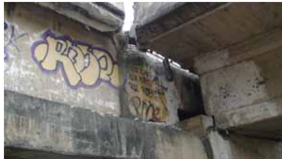
Figure 50. Photo. Interior face of westbound ramp to Llacolen bridge at the river end.
