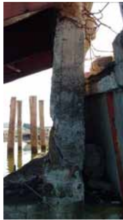
Figure 119. Photo. Shear crack in Tubul bridge.
