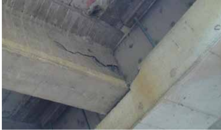
Figure 57. Photo. Horizontal crack in web of end girders at west end of Llacolen bridge.
