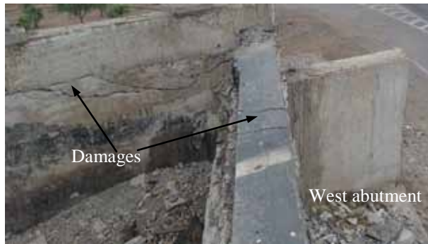
Figure 101. Photo. Back wall and wing wall damage at west abutment of Romero bridge.
