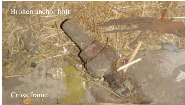
Figure 163. Photo. Anchor bolt failure (shear and pull out) on Route 5 pedestrian bridge.
