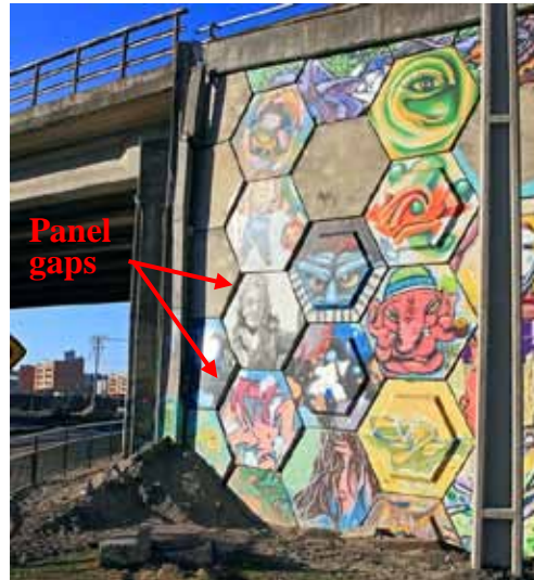
Figure 272. Photo. Differential settlement at wall site 28C.
