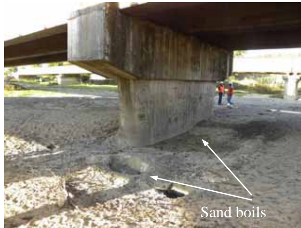
Figure 76. Photo. Sand boils close to pier under east Ramadillas bridge.
