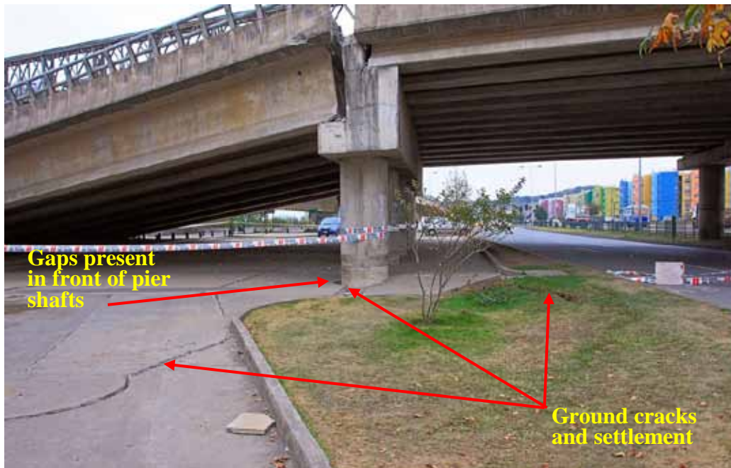
Figure 212. Photo. Settlement due to liquefaction-induced slope instability at northeast end of Llacolen bridge.
