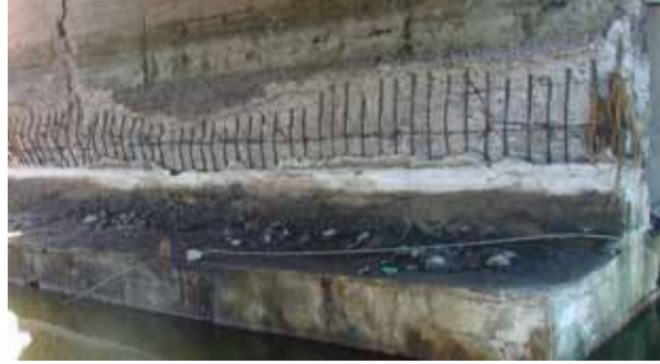
Figure 121. Photo. Spalling due to shear action and vertical crack in Tubul bridge.
