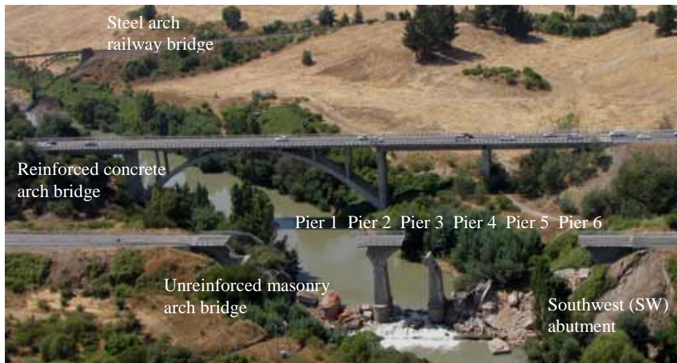
Figure 165. Photo. Collapse of masonry arch bridge at Claro River.
