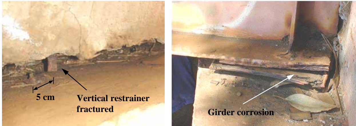
Figure 147. Photo. Damage on south abutment due to corrosion in Pichibudis bridge.
