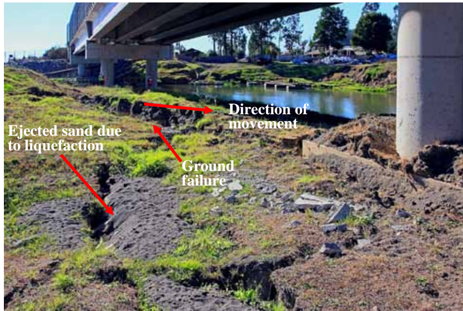
Figure 196. Photo. Ejected sand due to liquefaction and ground failure at La Mochita bridge.
