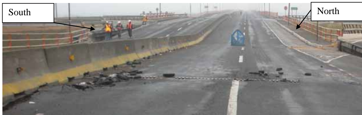
Figure 265. Photo. Wall settlement near Juan Pablo II bridge due to liquefaction-induced settlement.
