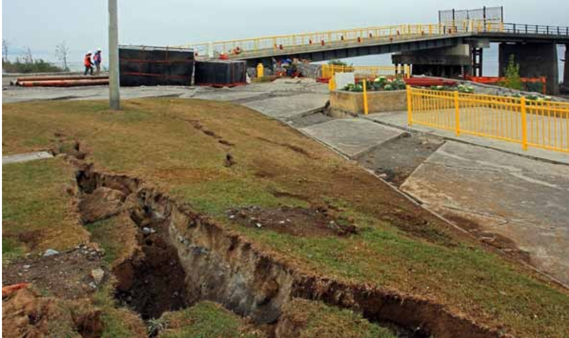
Figure 225. Photo. Ground failure near northeast abutment of old Biobío River bridge.
