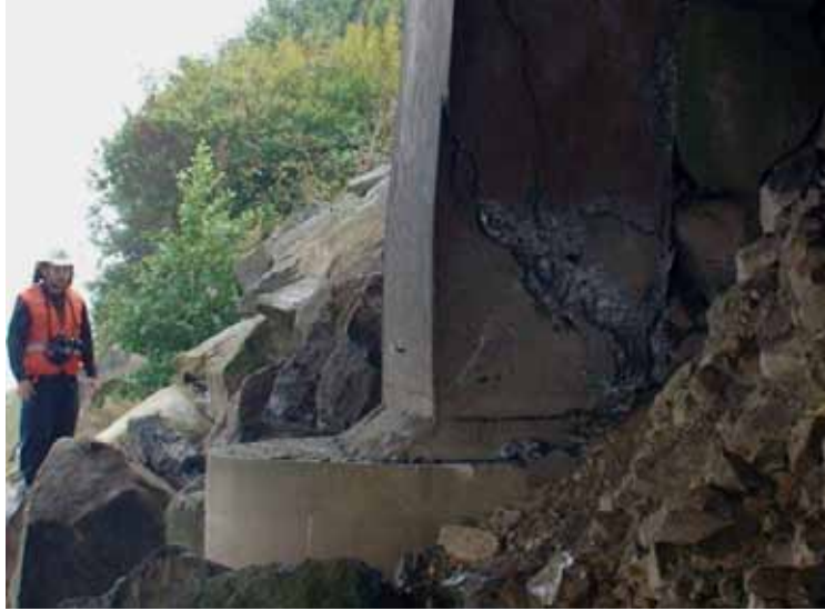
Figure 71. Photo. Shear failure in downstream column at northern end of Juan Pablo II bridge.
