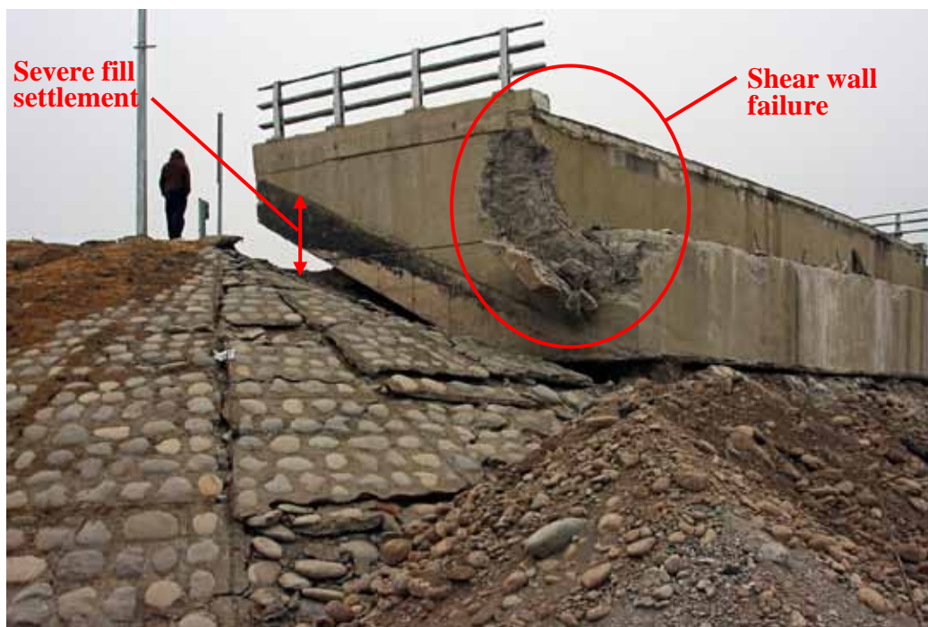
Figure 189. Photo. Fill slumping observed at Romero bridge.
