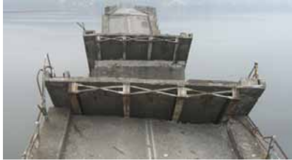
Figure 136. Photo. Unseated spans in Biobío River bridge.
