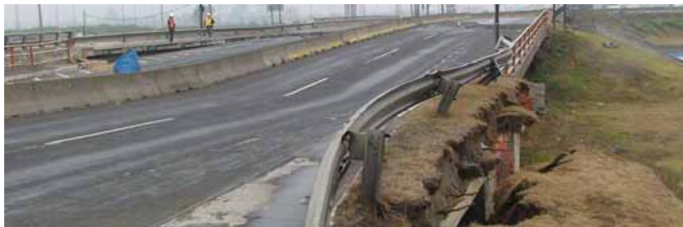
Figure 61. Photo. Northeast view of northern approach to Juan Pablo II bridge, facing away from Biobío River.
