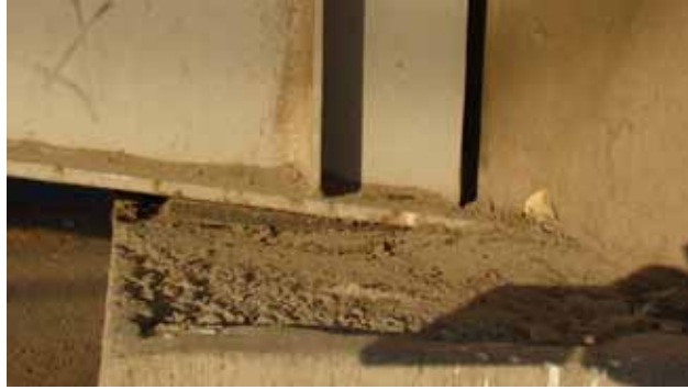
Figure 161. Photo. Steel girder on neoprene pad at abutment of Route 5 pedestrian bridge.
