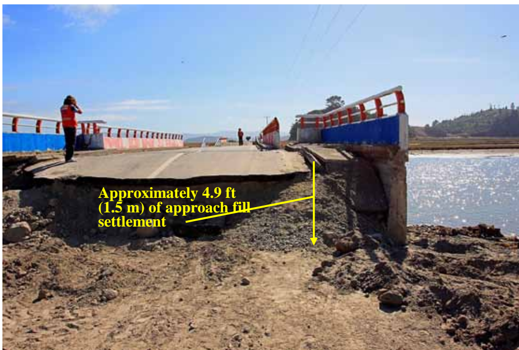
Figure 233. Photo. Southeast approach fill damage at Raqui 2 bridge.
