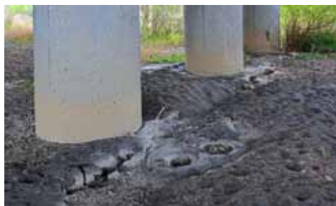
Figure 55. Photo. Sand boils near columns at west end of Llacolen bridge.
