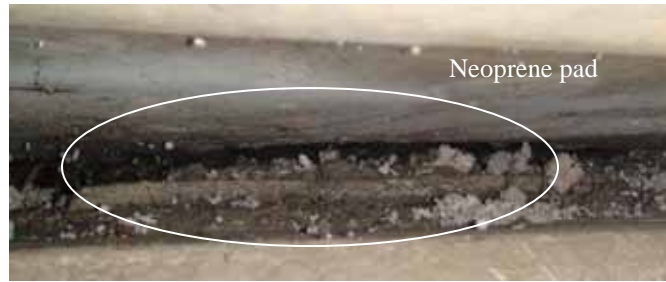
Figure 53. Photo. Neoprene pad degradation on westbound ramp to Llacolen bridge.
