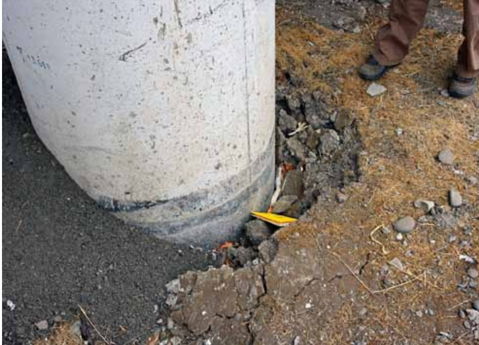
Figure 186. Photo. Interior pier of Chada structure with 5.8- to 7.8-inch (150- to 200-mm) gap in soil transverse to bridge centerline.
