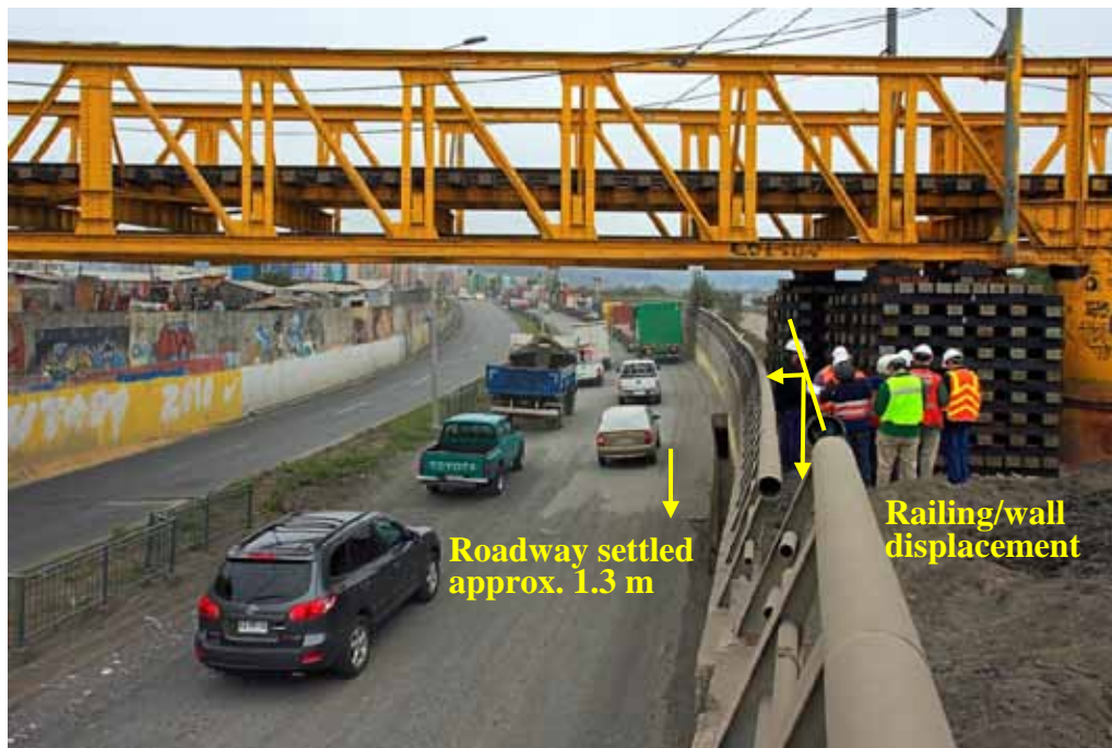
Figure 216. Photo. Wall settlement due to slope movement and instability caused by liquefaction at northwest end of Chepe railroad bridge.
