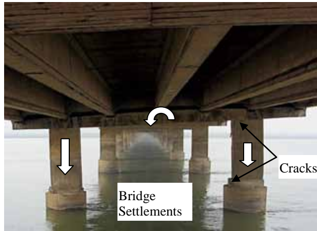
Figure 67. Photo. Differential settlement underneath first span over water at northern end of Juan Pablo II bridge.
