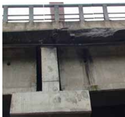
Figure 56. Photo. Spalling in deck slab at west end of Llacolen bridge.
