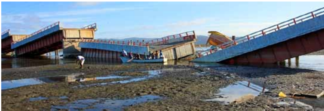
Figure 241. Photo. Tubul bridge collapsed spans and substructure.
