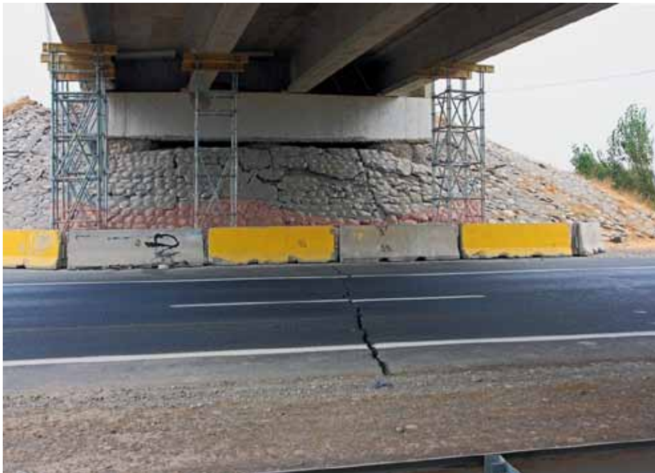
Figure 187. Photo. East abutment of Chada structure showing large pavement crack directly below bridge centerline.
