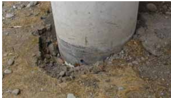
Figure 39. Photo. Soil separation from column of Chada bridge.
