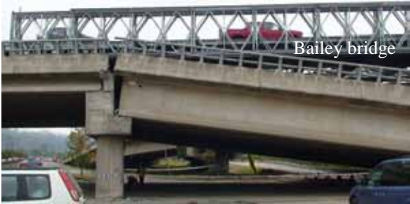
Figure 43. Photo. Unseated simply supported span in eastern approach to Llacolen bridge.
