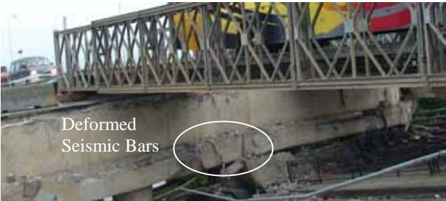
Figure 44. Photo. Abutment at unseated end of span in eastern approach to Llacolen bridge.
