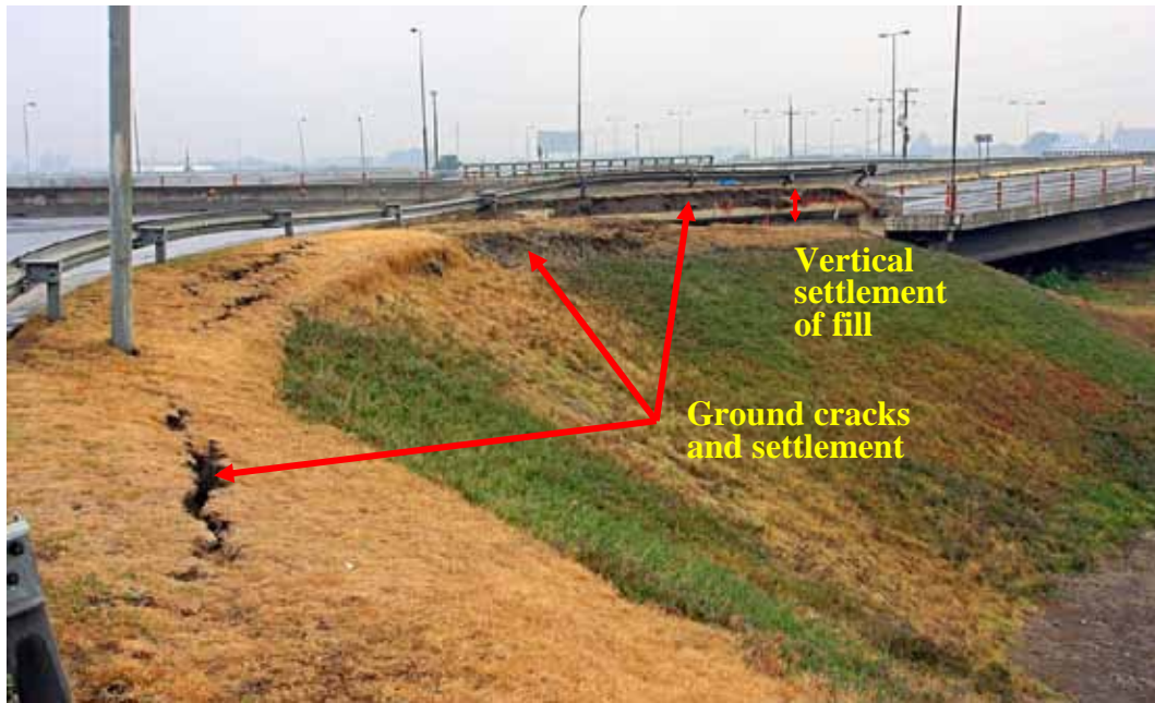
Figure 200. Photo. Ramps at Juan Pablo II bridge where existing ground was improved with DDC.
