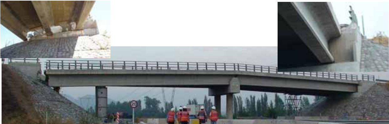
Figure 41. Photo. Las Mercedes bridge and girder unseating at abutments.
