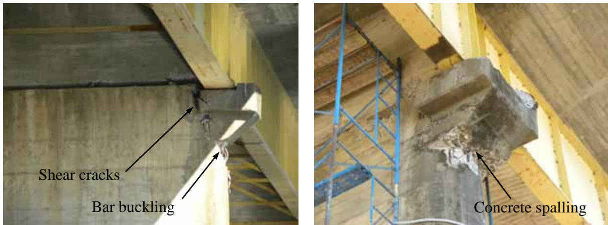
Figure 159. Photo. Damage to girder supports of Itata River bridge.
