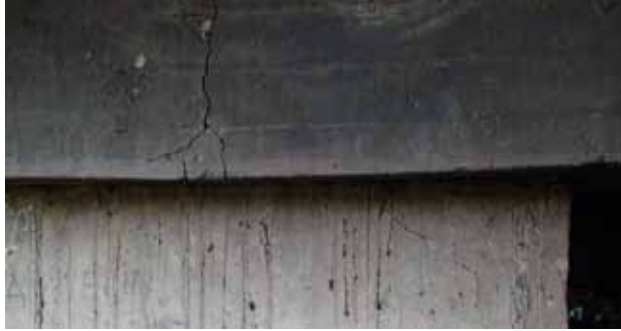
Figure 66. Photo. Cracks on far side of undamaged column under approach to Juan Pablo II bridge.
