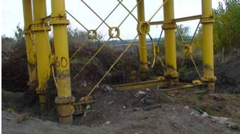
Figure 179. Photo. Ruptured cross bracing at south end of Chepe railroad bridge.
