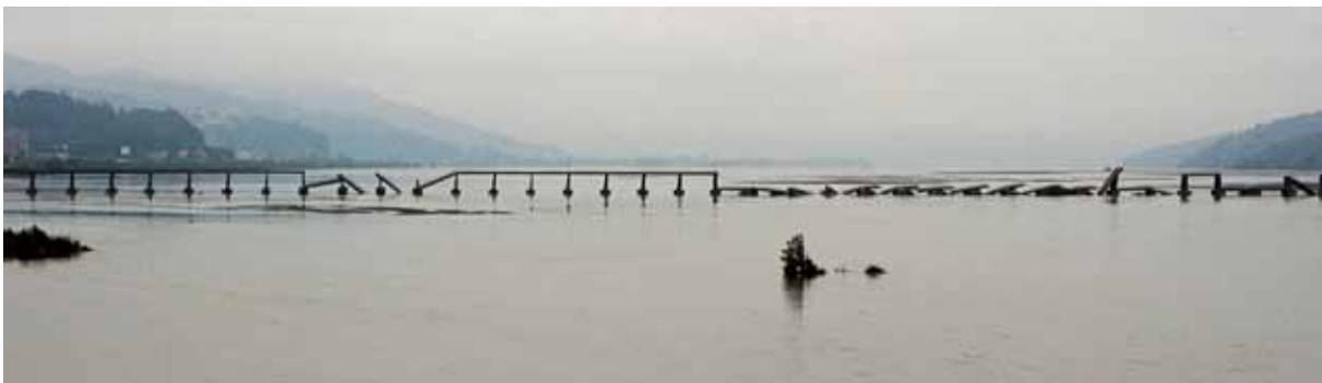
Figure 138. Photo. Collapsed spans and piers of Biobío River bridge.
