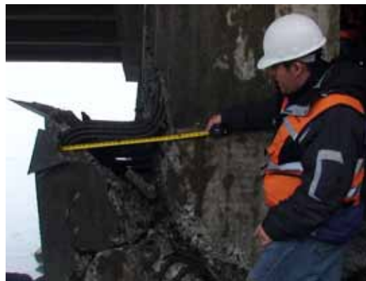
Figure 69. Photo. Front face of failure plane at northern end of Juan Pablo II bridge.
