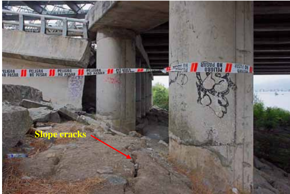
Figure 214. Photo. Lateral ground and foundation movement at interior pier and fallen span at northeast end of Llacolen bridge.
