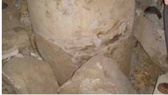
Figure 46. Photo. Flexural cracks at the level of rip rap on eastern approach to Llacolen bridge.
