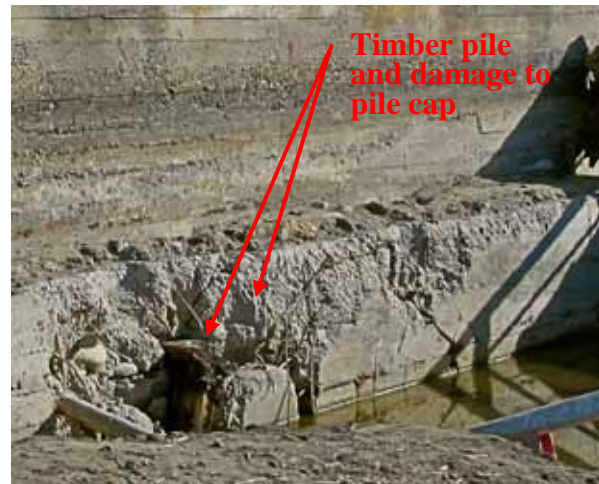
Figure 239. Photo. Close-up of exposed pile and pile cap damage on south abutment of Tubul bridge.
