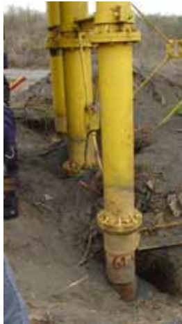
Figure 180. Photo. Fractured steel piles at south end of Chepe railroad bridge.
