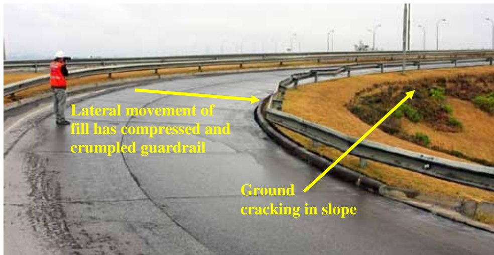
Figure 201. Photo. Lateral movement of fill in ramps at Juan Pablo II bridge.
