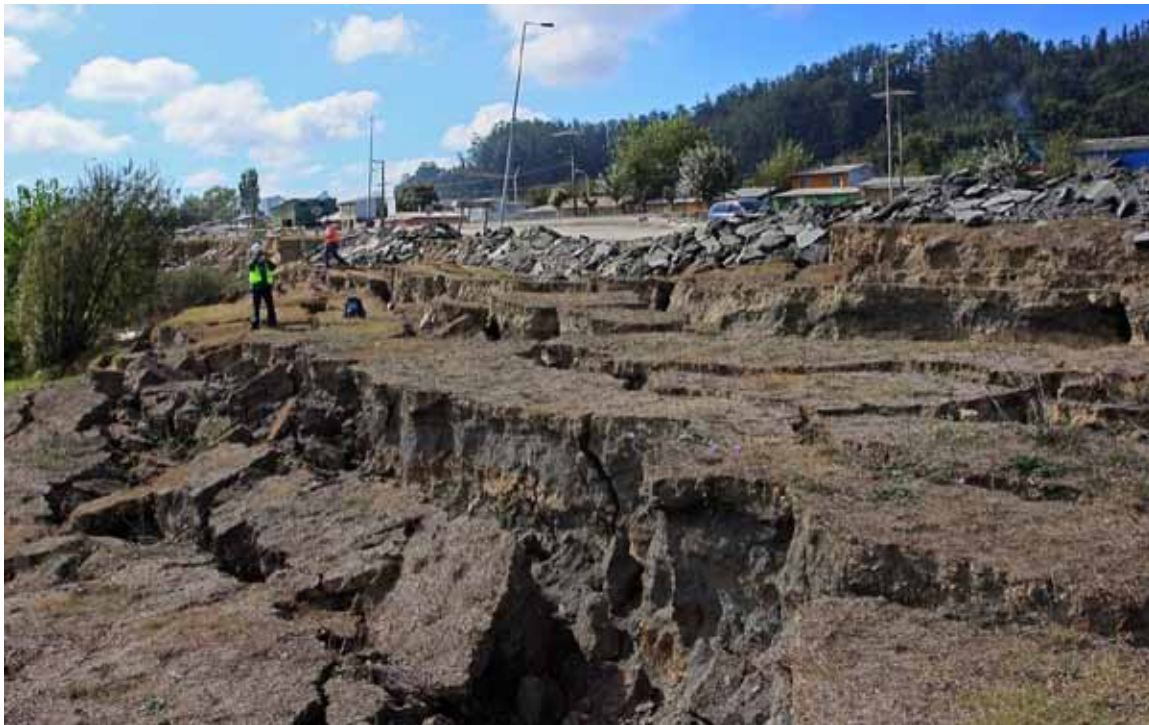
Figure 227. Photo. Ground failure of north approach fill for La Mochita bridge.
