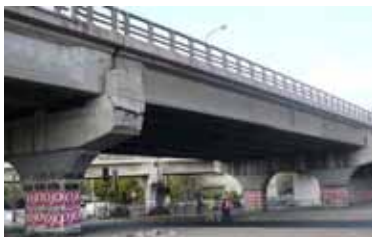
Figure 30. Photo. Shear key damage at intermediate bents of westbound Independencia bridge.
