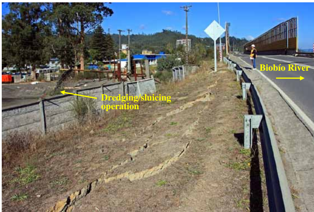
Figure 229. Photo. La Mochita bridge north approach fill and edge of dredging pit.
