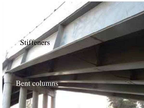
Figure 108. Photo. Stiffeners on Quilicura railway overcrossing.
