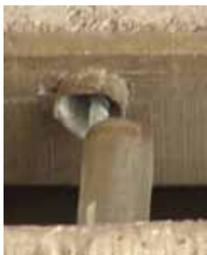
Figure 28. Photo. Displaced seismic bar on westbound Independencia bridge.
