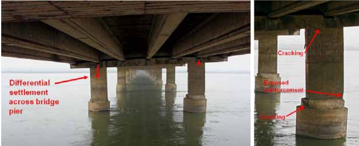
Figure 221. Photo. Liquefaction-induced differential settlement of mainline pier foundations supporting Juan Pablo II bridge.
