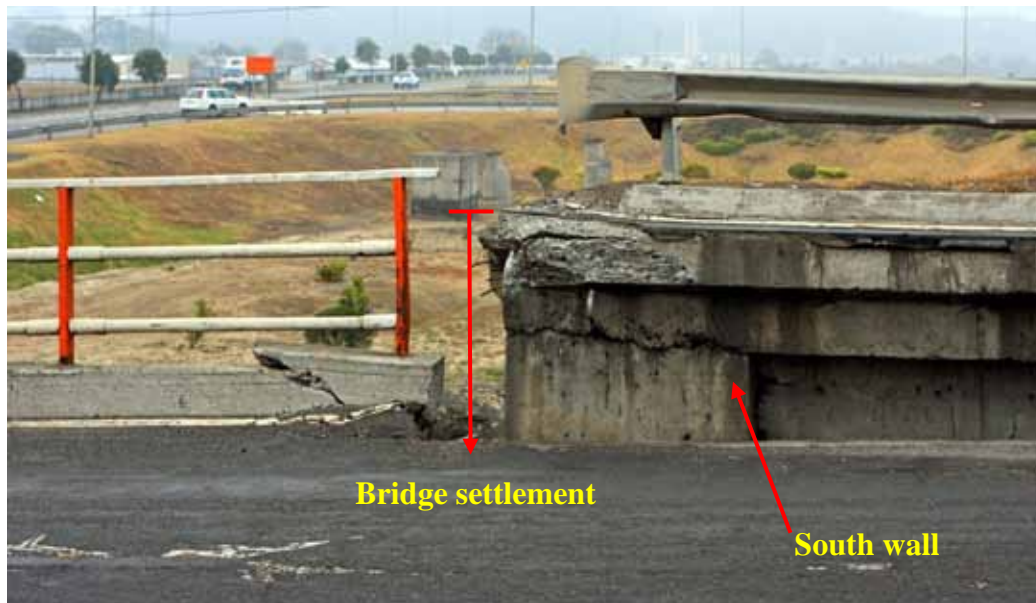
Figure 218. Photo. Close-up of settlement of approach structure for Juan Pablo II bridge.
