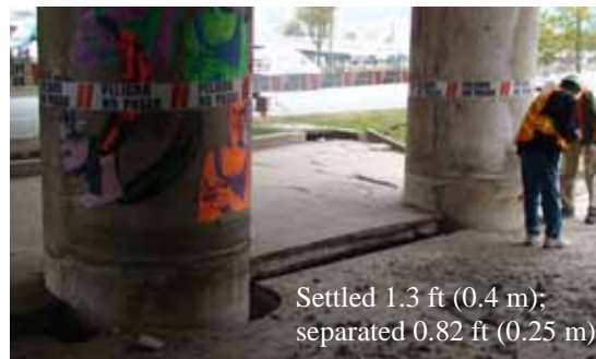
Figure 48. Photo. Ground settlement and lateral movement of eastern approach to Llacolen bridge.
