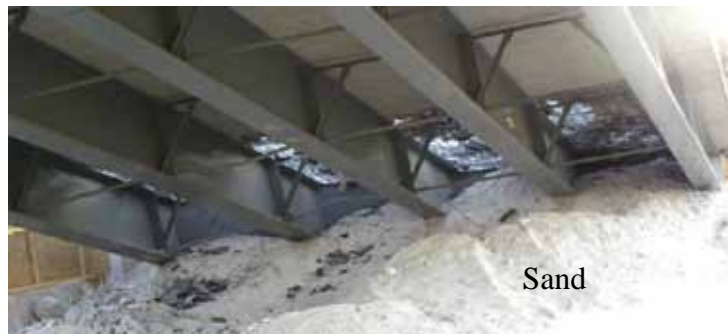
Figure 111. Photo. West span of Quilicura railway overcrossing lowered onto sandbank.
