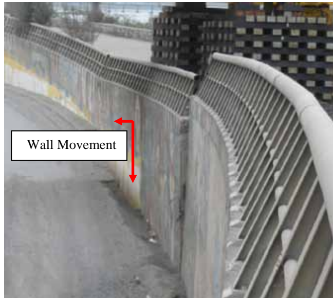
Figure 262. Photo. Wall movement near Chepe railroad bridge due to lateral spreading and settlement.
