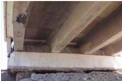
Figure 281. Photo. Exterior girder damage at Chada bridge, no diaphragms.
