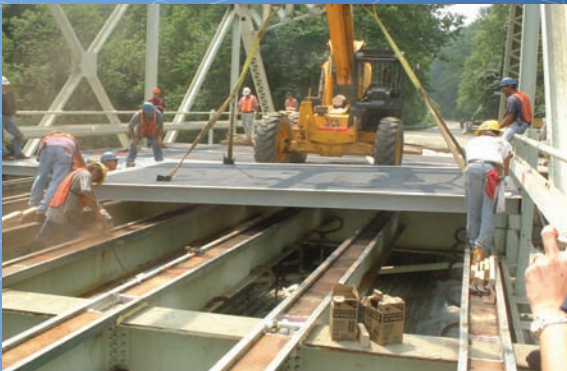
Placement of Fiber Reinforced Polymer (FRP) deck panels on steel girders of a 125-foot through-truss bridge at MD Route 24, north of Baltimore, near Rock Creek State Park.
