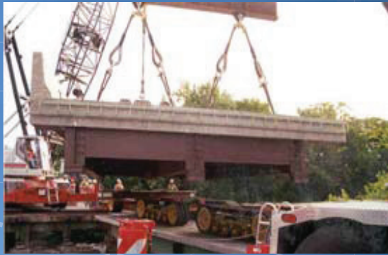
I-95 over the James River in Virginia was completed in October 2009. Preconstructed composite units (PCUs) were lifted into place during nighttime closures from 7:00 pm to 6:00 am the next day.
