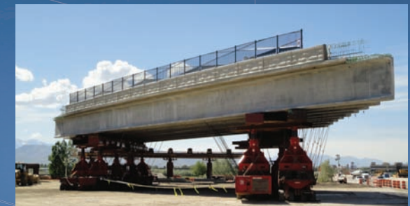
Self-propelled modular transporters (SPMTs) move bridge superstructure into place in hours, minimizing traffic disruption.
