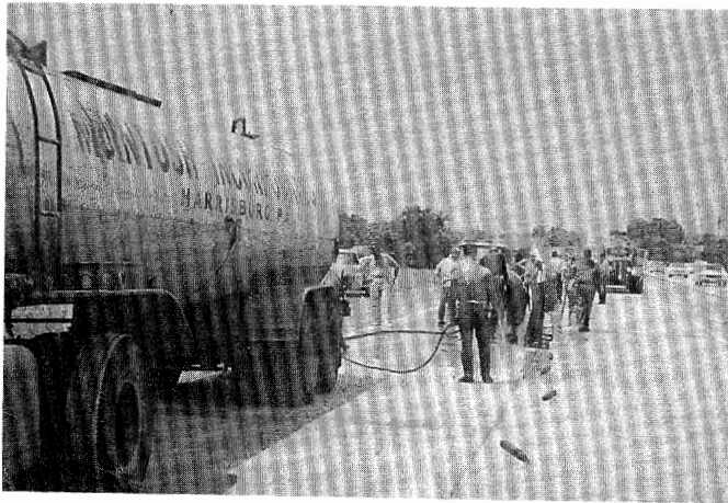
This photo depicts the process of raising a slab to its original grade with a high-softening-point asphalt cement.
