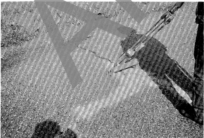
Hot air blasting (using a heat lance) dries the crack before sealing. The maintenance technician should take care not to burn the asphalt around the crack by moving the heat lance too slowly.
