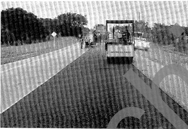
The Novachip mix is rolled immediately after placement. Two 9Mg rollers were used for a total of four passes.
