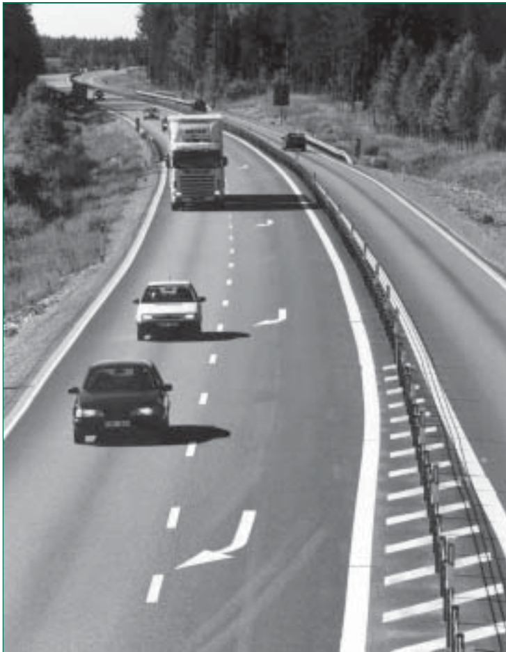
Figure 3. Sweden improved safety on many two-lane rural roadways by converting them to 2+1 facilities with alternating passing lanes.
