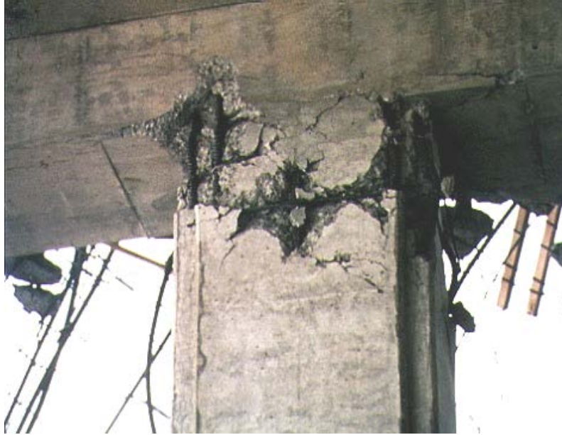
Figure 6-1 Poorly Confined Column in 1971 San Fernando Earthquake
