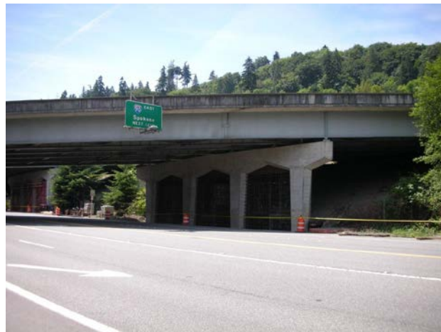
(b) Steel girders on bearings
