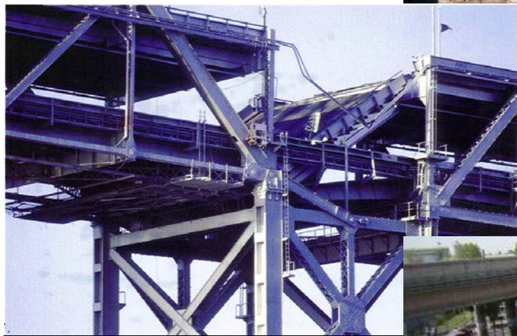
San Francisco Oakland Bay Bridge, Loma Prieta, 1989
