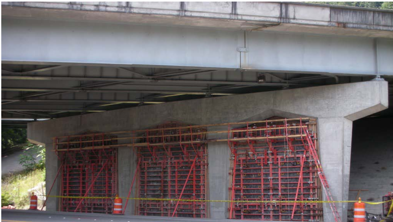
Figure 10-10(f) Infilled Walls for Concrete Piers (top) and Installation on West Lake Sammish Parkway, I-90 Retrofit, photo L.M. Marsh (bottom)
