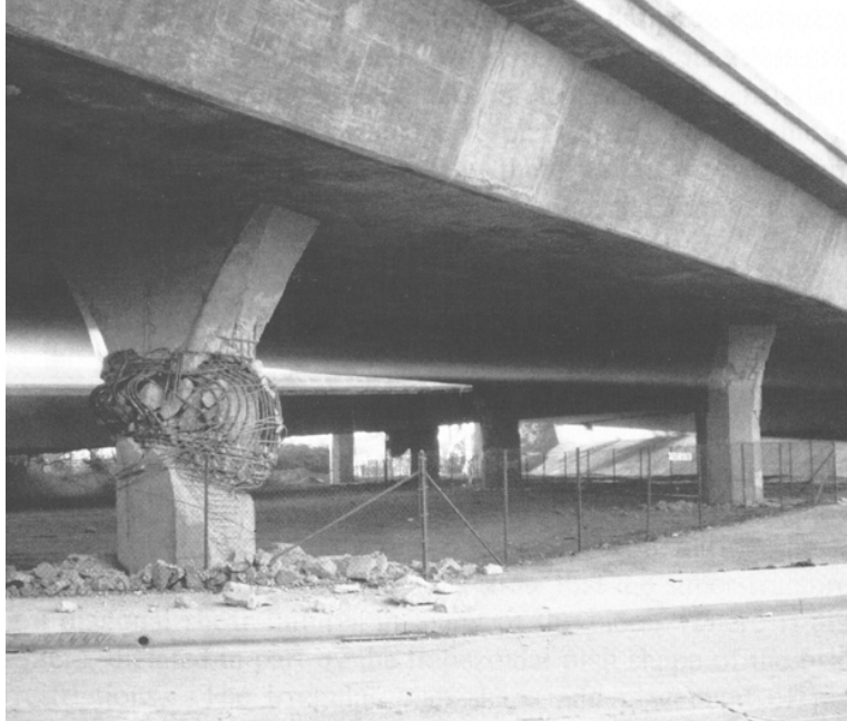
Figure 6-14 Damage to Integral Flared Columns in the 1994 Northridge Earthquake (Nada, Sanders, and Saiidi, 2003)
