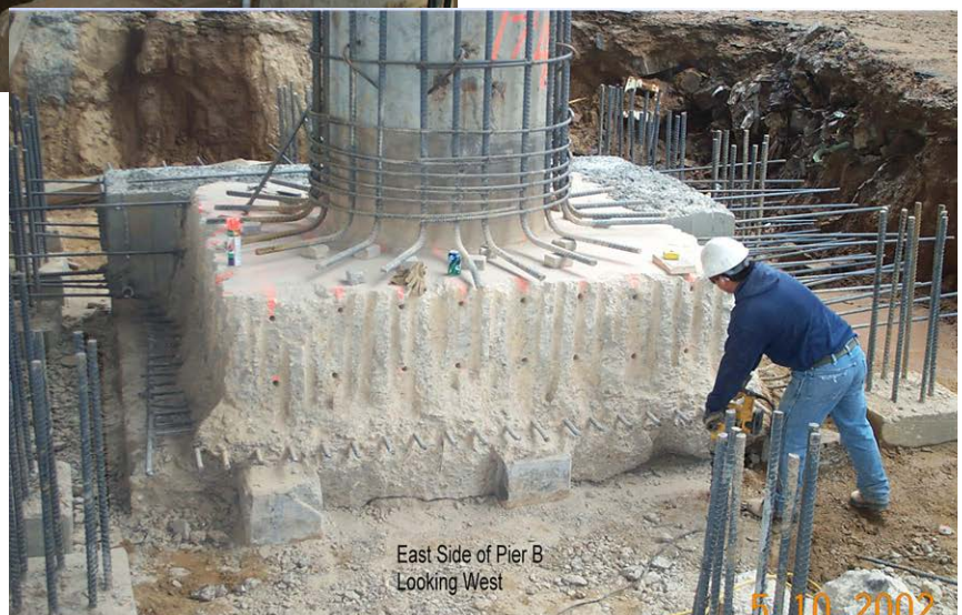
Figure 10-10(g) Footing Overlay with Piled Extension (top) and Installation on Hernando-Desoto Bridge, I-40 Retrofit, photo R.A. Imbsen (center and bottom)
