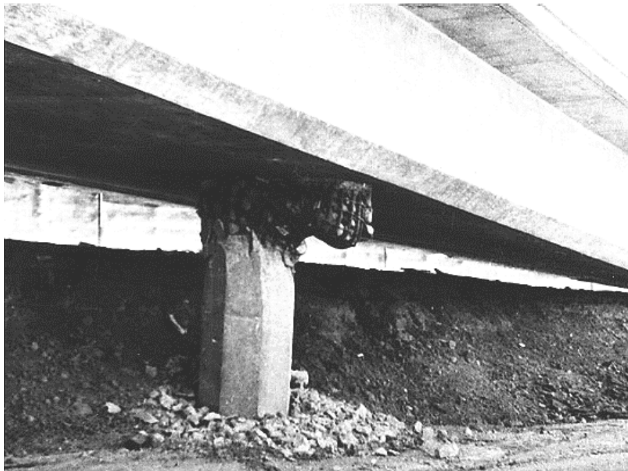
Figure 6-7 Shear Failure of a Column in the 1971 San Fernando Earthquake
