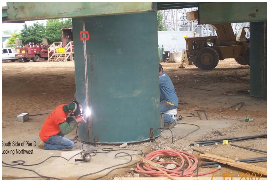
Figure 10-10(e) Steel Jackets for Concrete Columns (top) and Installation on Hernando Desoto Bridge, I-40 Retrofit, photo R.A. Imbsen (bottom)
