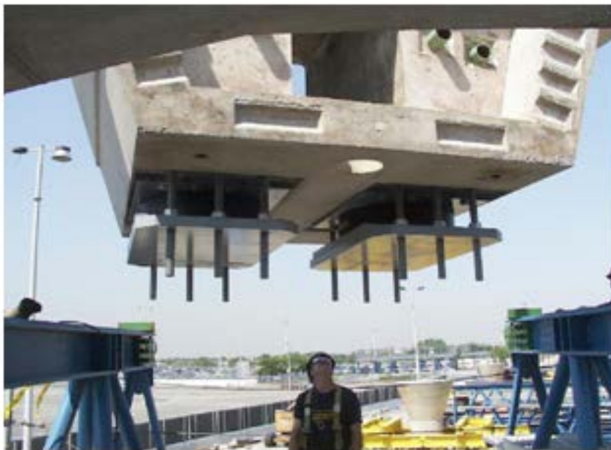
Figure 9-8 Lead-Rubber Isolators Being Installed in the JFK Airport Light Rail Viaduct, NY
